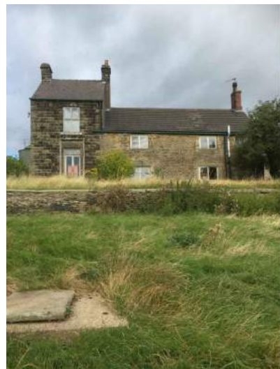
8. Facing north, view of the original farm house and associated extension. Cesspit is in the foreground.
