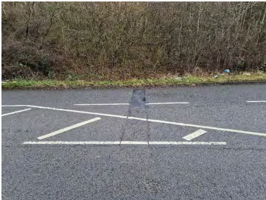
Photo 40 – Failed reinstatement to north of junction with Ashroyds Way on Ryecroft Bank at start of right turn lane.
