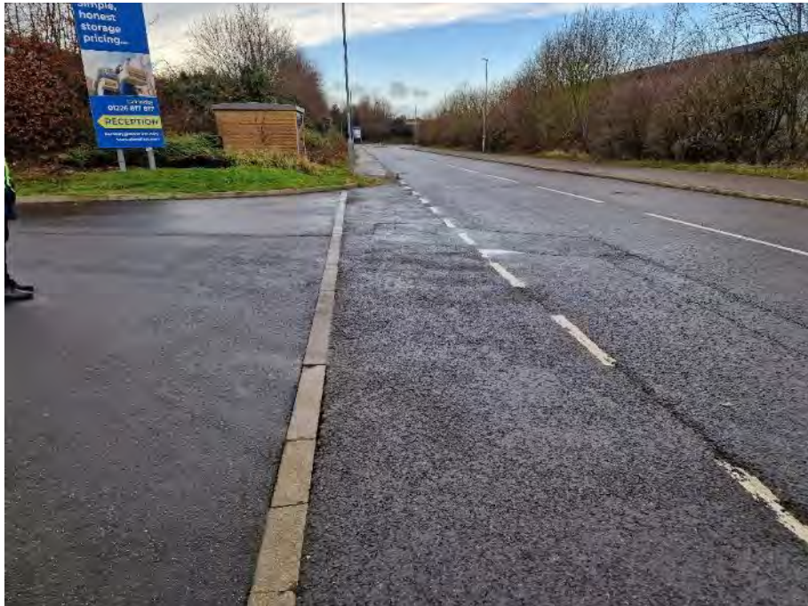
Photo 57 – Damaged channel blocks across Plot 4B entrance.
