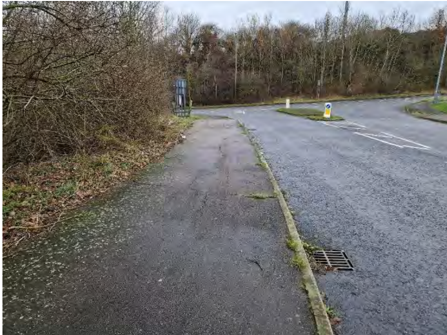
Photo 34 - View along northern footway – depression in footway along near entire length.
