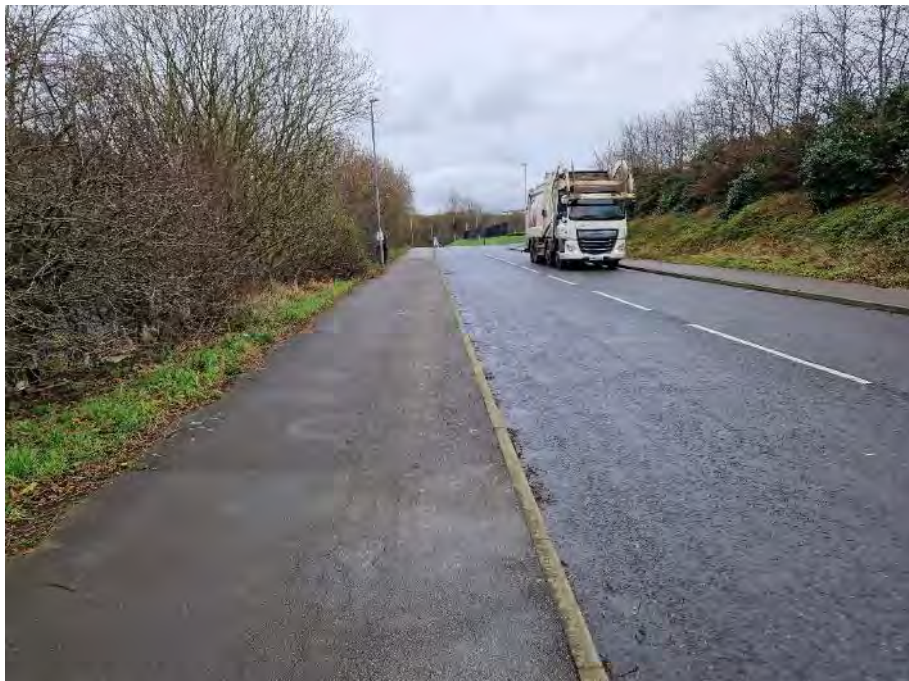
Photo 24 - View along northern footway – depression in footway along near entire length.
