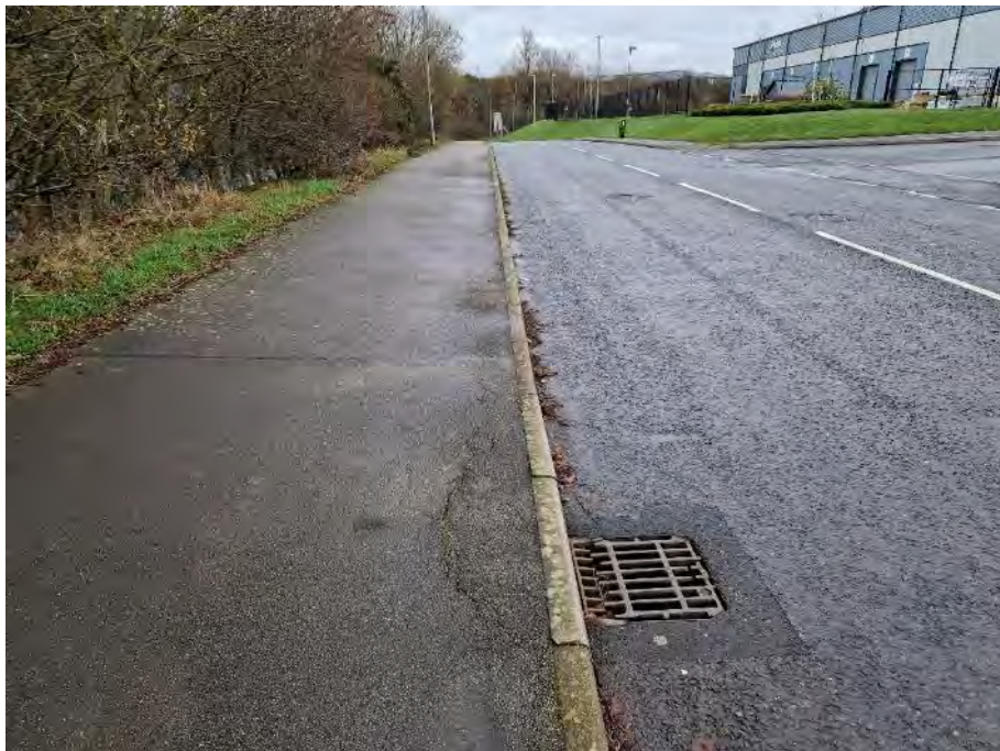
Photo 28 – Depression to rear of kerb.
