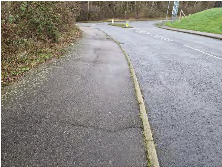
Photo 33 - View along northern footway – depression in footway along near entire length.
