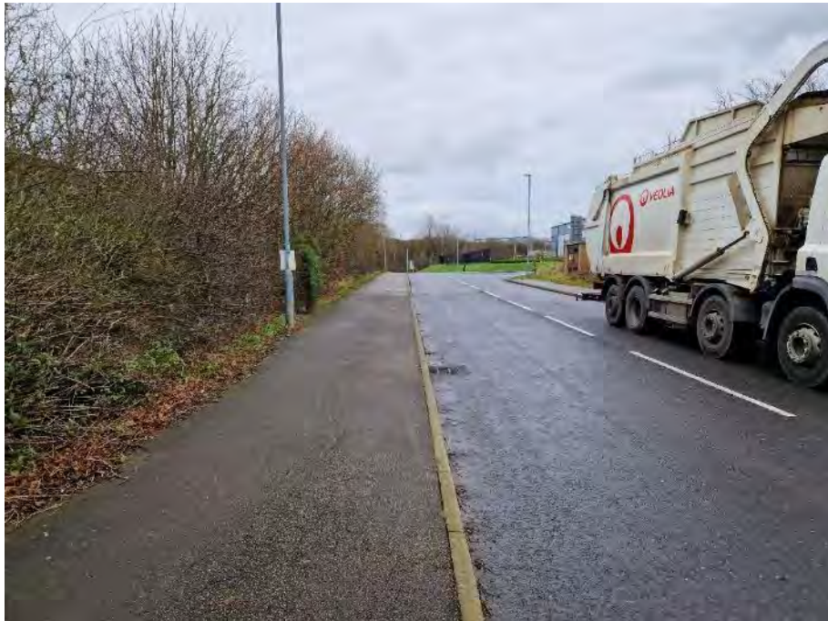
Photo 25 - View along northern footway – depression in footway along near entire length.
