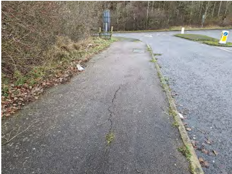
Photo 35 - View along northern footway – depression in footway along near entire length.
