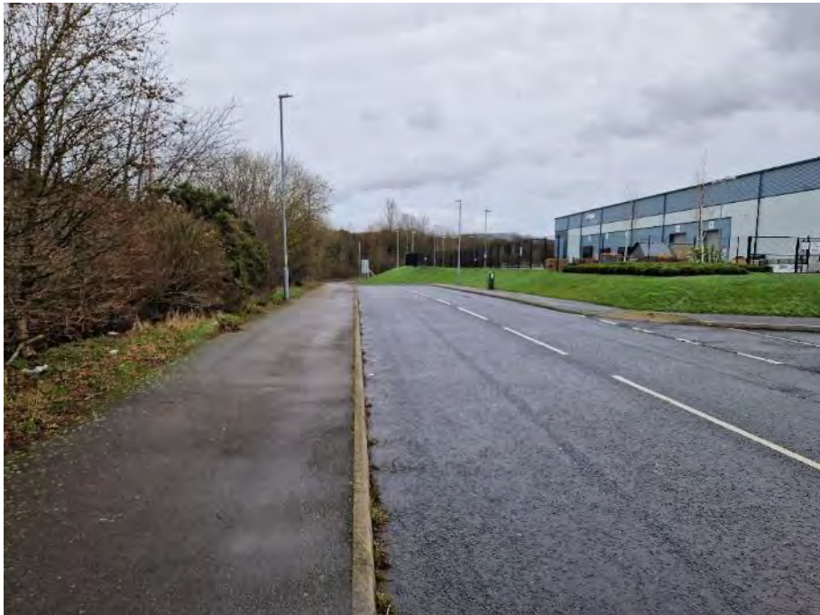
Photo 29 - View along northern footway – depression in footway along near entire length.
