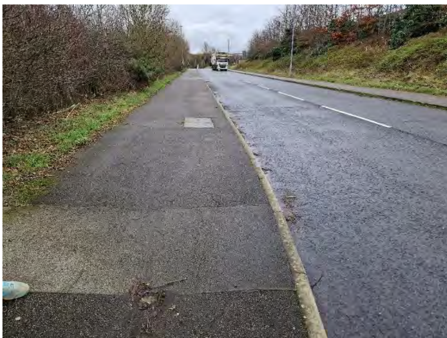
Photo 22 – View along northern footway – depression in footway along near entire length.
