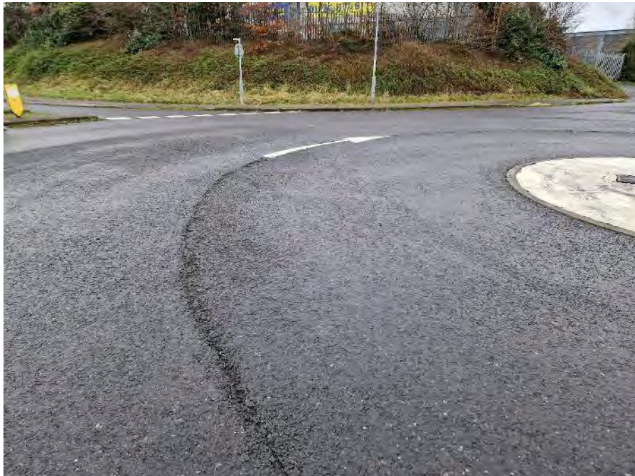
Photo 19 – View across roundabout – looking at the joint in surfacing.
