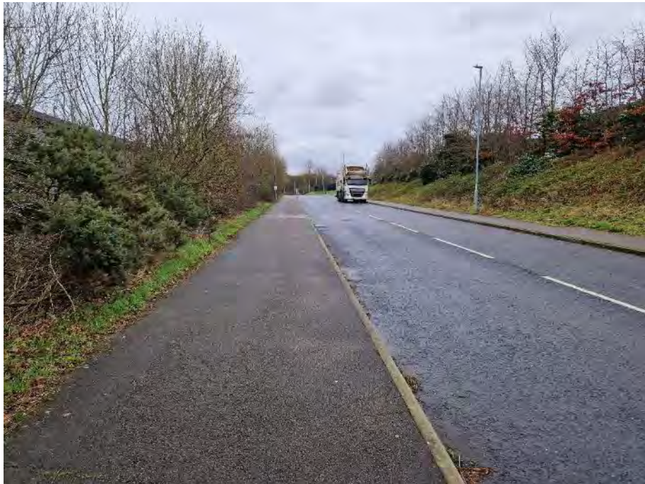
Photo 23 - View along northern footway – depression in footway along near entire length.
