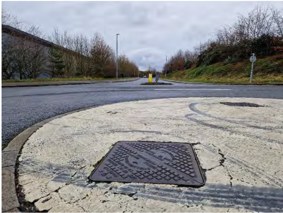
Photo 17 – Depression in centre of roundabout
