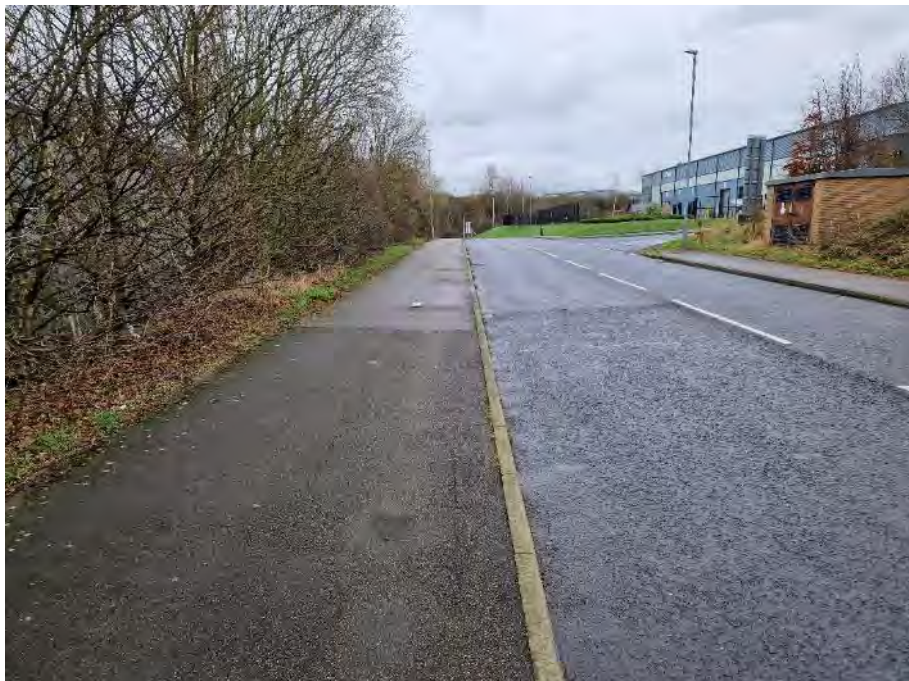
Photo 26 - View along northern footway – depression in footway along near entire length.
