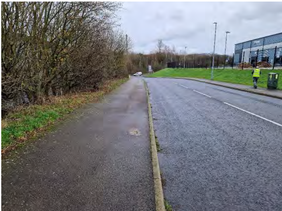
Photo 30 - View along northern footway – depression in footway along near entire length.
