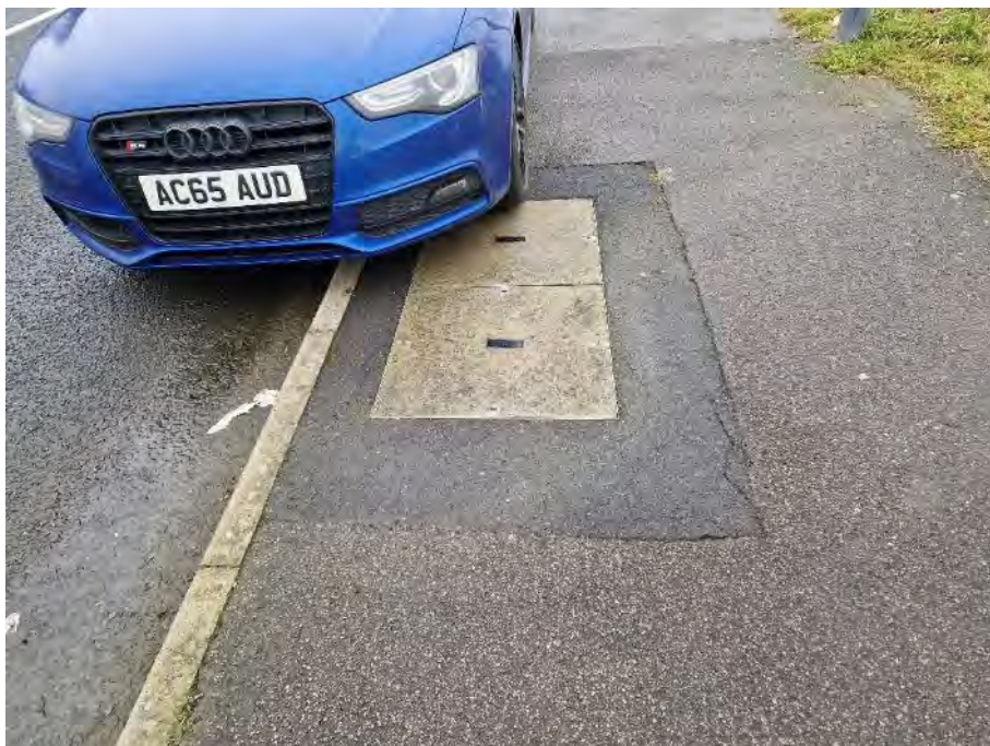
Photo 8 – BT chamber in footway.
