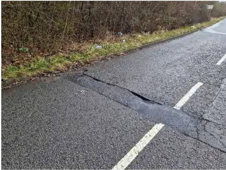
Photo 41 - Failed reinstatement to north of junction with Ashroyds Way on Ryecroft Bank at start of right turn lane.
