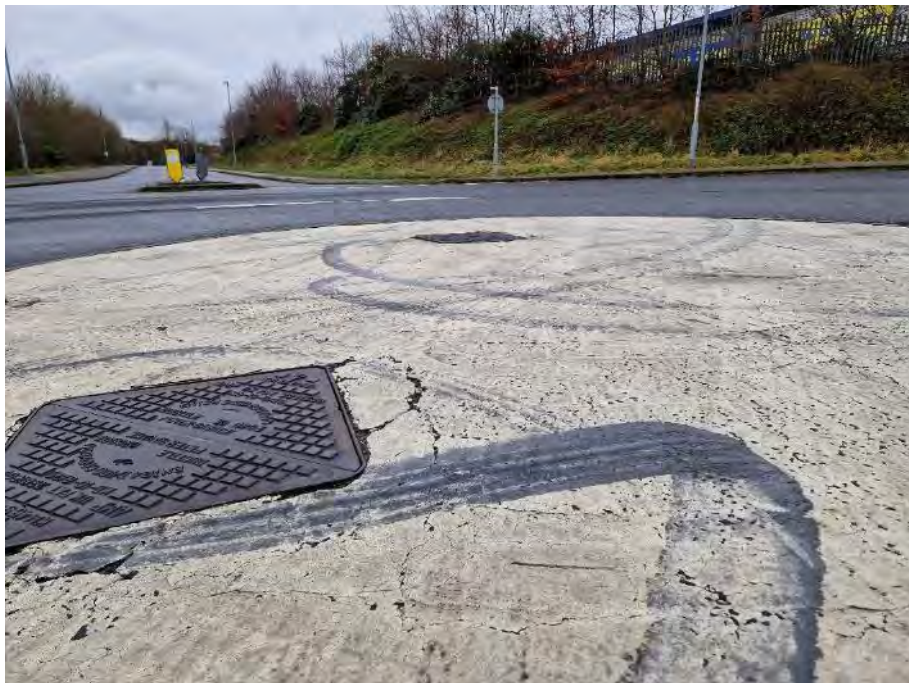
Photo 18 – Depression in centre of roundabout
