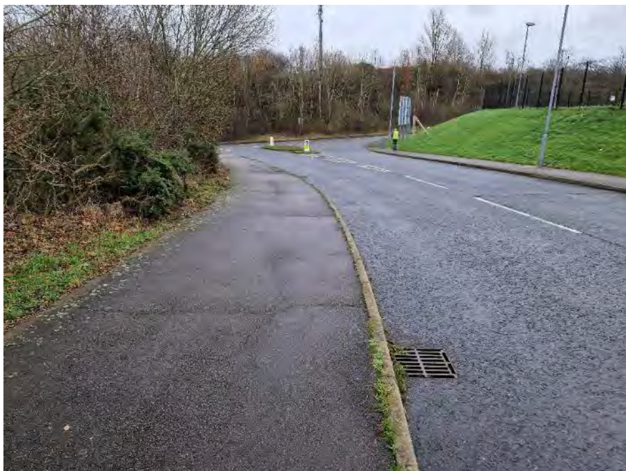
Photo 32 - View along northern footway – depression in footway along near entire length.
