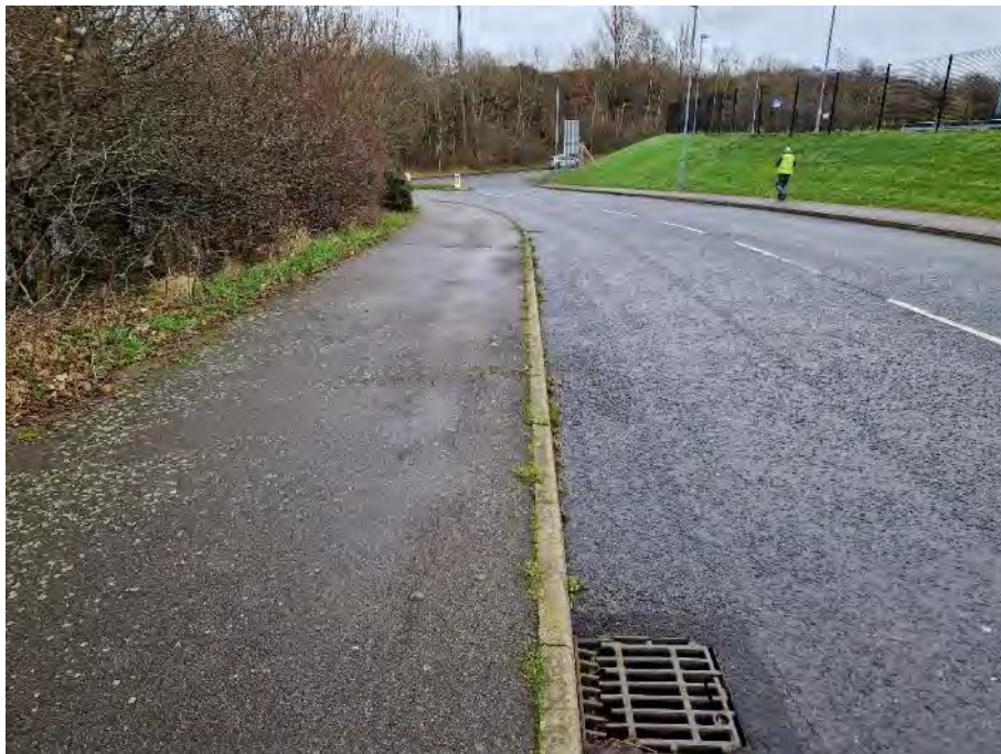
Photo 31 - View along northern footway – depression in footway along near entire length.
