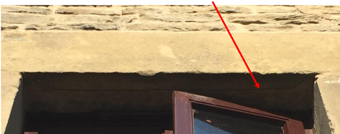
Examples of cill and head with retrospective channels cut try and prevent water penetration.
