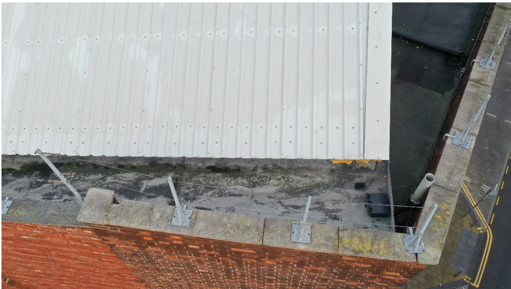
Fig 11. The parapet is capped with concrete copings, some of which are cracked/broken and some dislodged.
