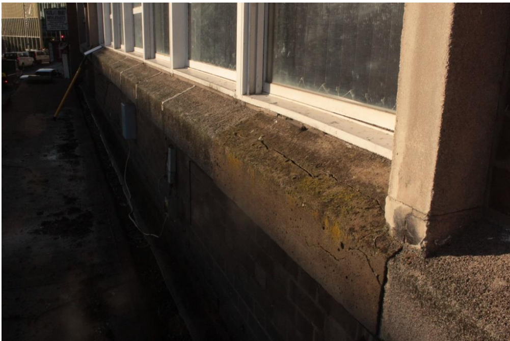
Fig 23. Repair of a cill section (poorly executed and now cracking) and spalling at the cill joints which has been temporarily covered with flashband.
