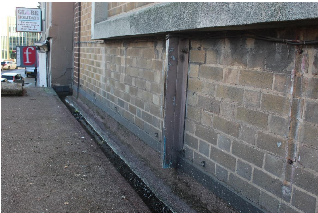
Fig 30. One of the timber posts fixed back to the brickwork with an angle iron bracket beneath the first floor windows.
