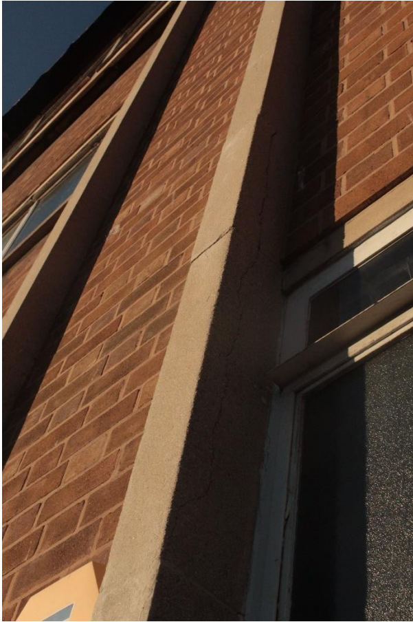
Fig 24. Cracks extending up the side of two units forming one of the concrete mullions.
