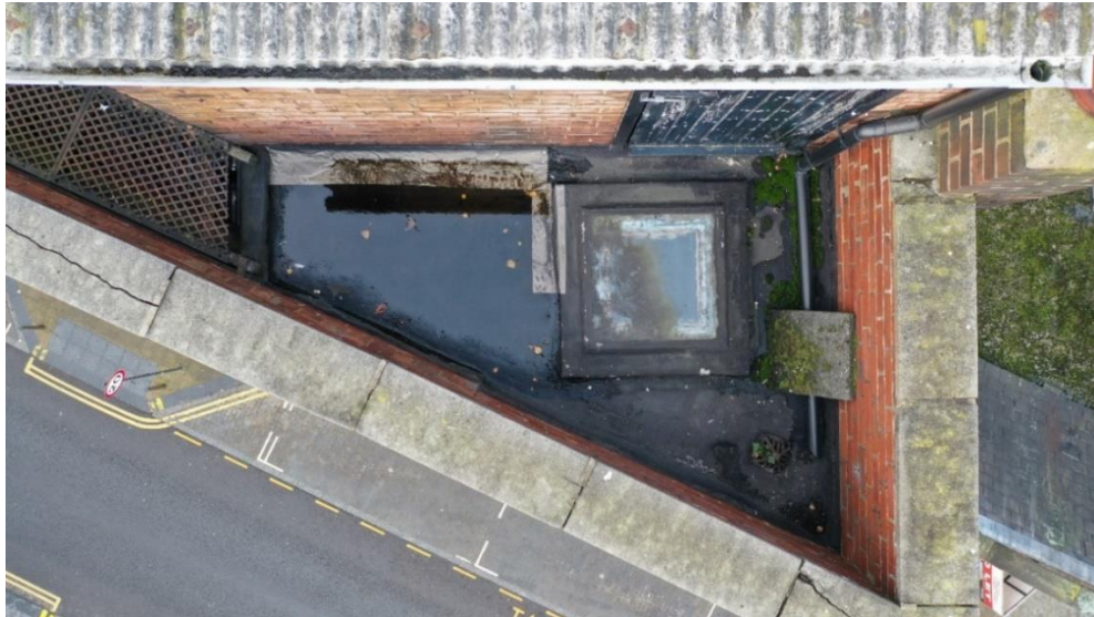
Fig 16. The small triangular flat roof in front of the door into the lean-to structure at the north-eastern corner of the roof.
