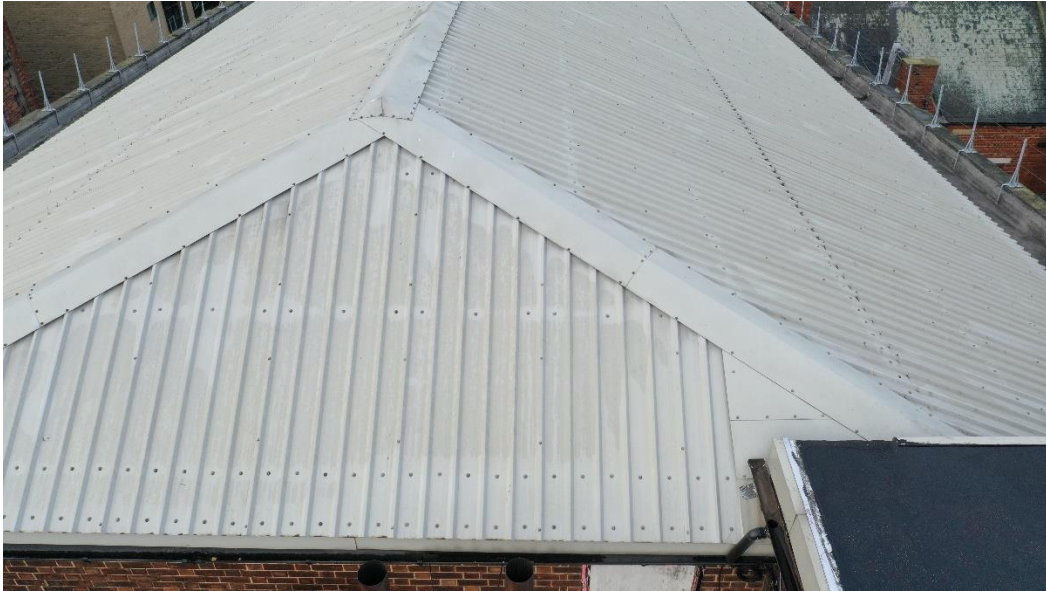
Fig 10. The east facing pitch empties into a black plastic gutter and thereby via a black plastic downpipe onto the flat roof above the Eldon Street entrance.
