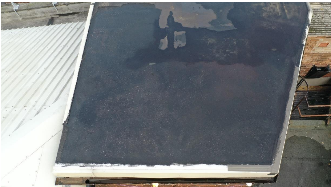
Fig 14. Rainwater ponding in the southern gutter of the stair enclosure (bottom of photo).
