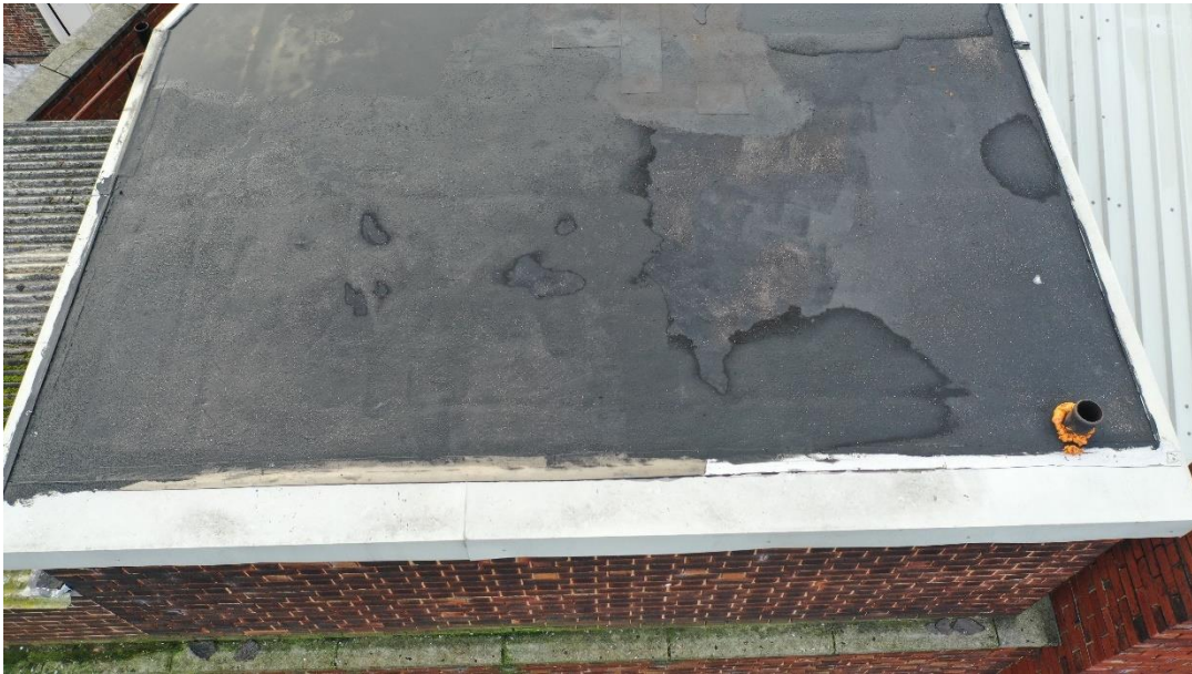
Fig 13. The flat roof over the stair enclosure is finished with black bitumen-based roofing felt which has been patch repaired and finished with bitumen paint.
