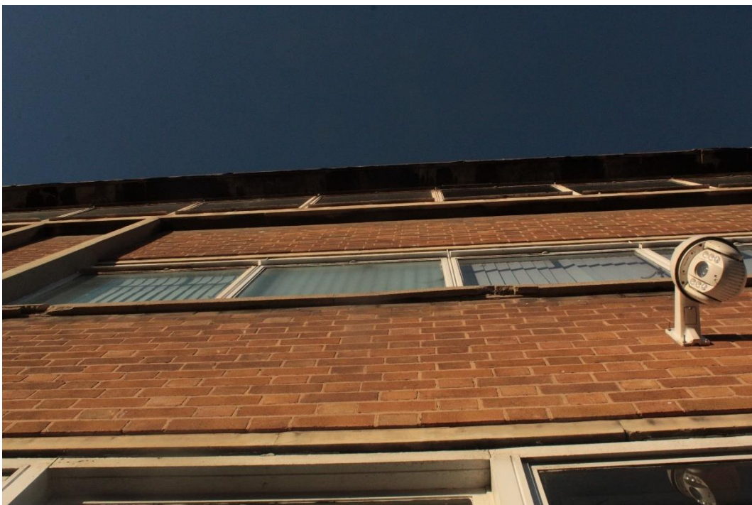
Fig 27. Cracking and damage extending almost the full length of one of the second floor window cill units. Far left similar cracking and damage along the same cill.
