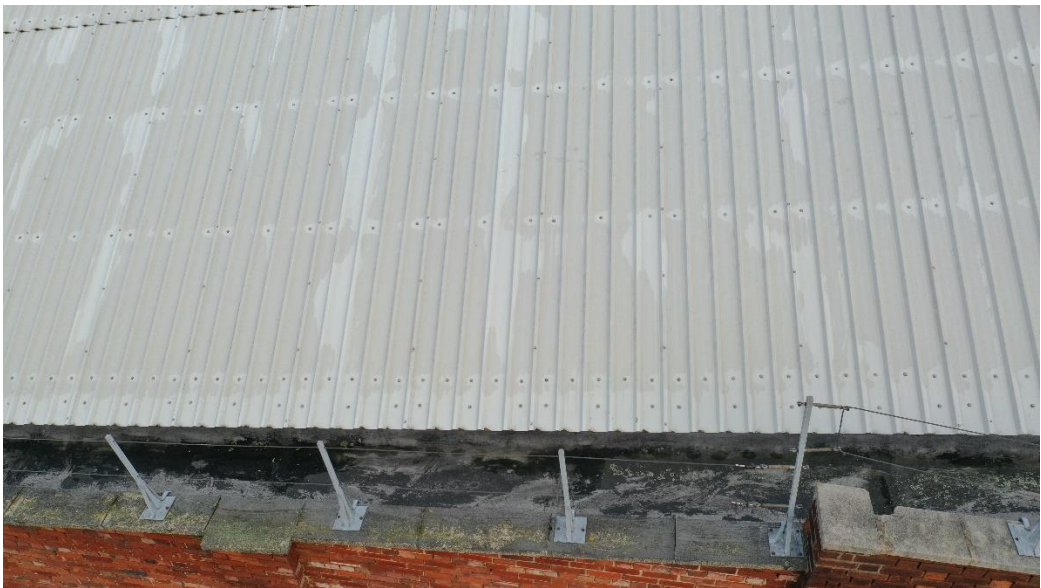
Fig 09. There is creep and splitting visible (in the dark area immediately above the projecting coping far left) in the bitumen felt lining the parapet gutter, throughout the gutter length.
