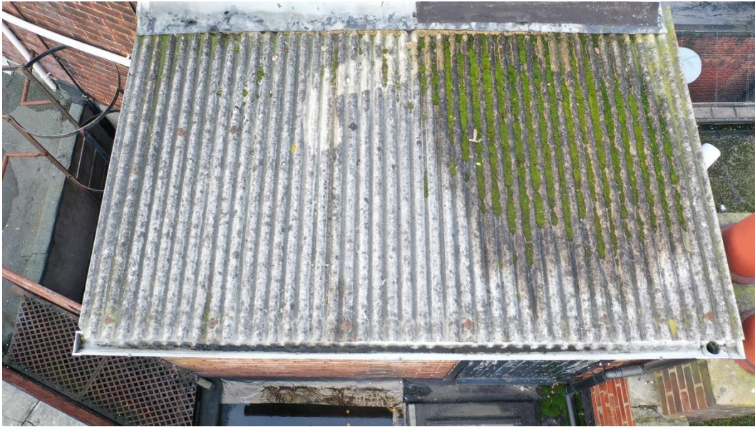
Fig 15. The small lean-to structure abutting the eastern (front) elevation of the stair enclosure which is finished with profiled asbestos cement sheeting.
