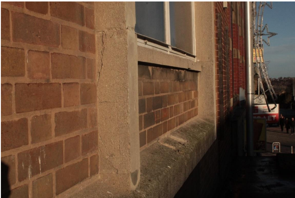
Fig 21. Cracks to the first-floor window cill indicating corroded embedded steel reinforcing. Spalling at (and repair of) the joint in the concrete lintel and corresponding hairline cracks up the side of the concrete mullion. Note also, the hairline crack visible in the adjoining vertical section of the concrete 'frame' beyond the window, above cill level.
