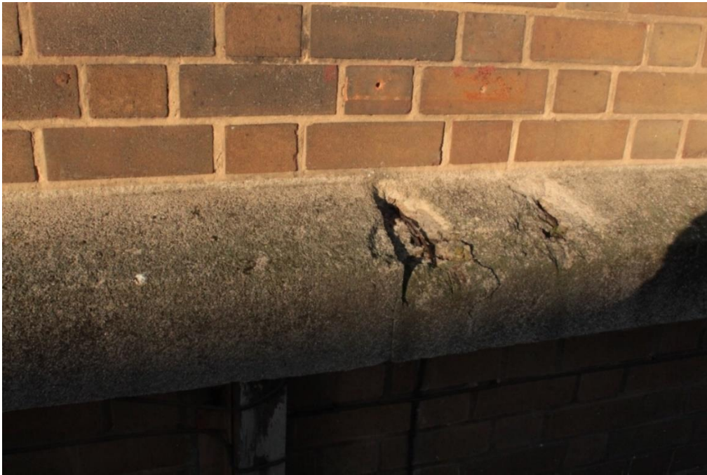
Fig 20. Concrete spalling which has exposed the shallow steel reinforcing bars in a number of places along the cill of the concrete 'frame'.
