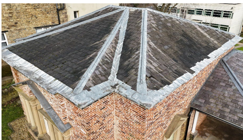
Existing Roof Coverings and Lead Apron Detail Prior to Stripping the South Slope
