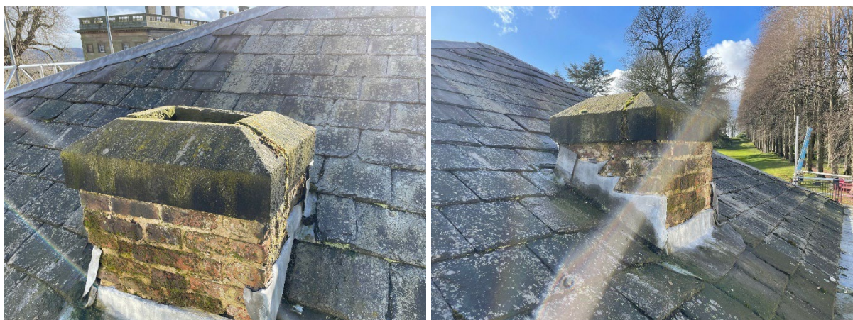
Existing Chimney Detail with Loose Flashings and Weathered Pointing
