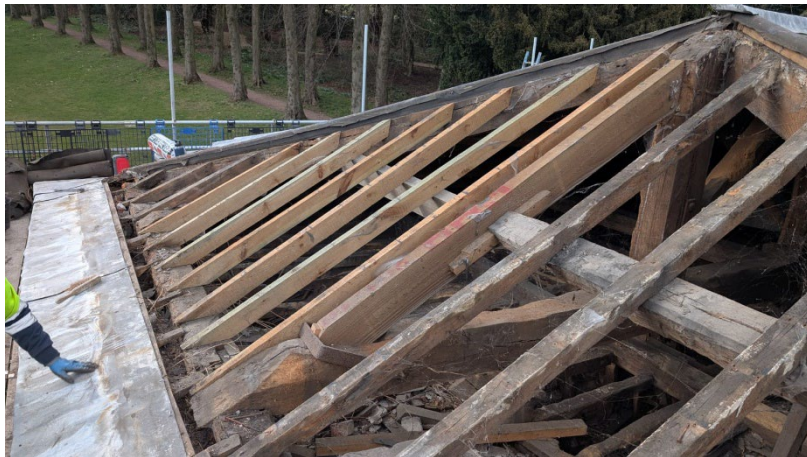
Existing roof structure to the south elevation where coverings have been stripped.
