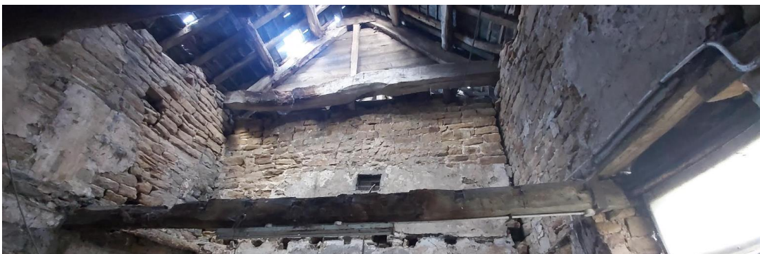
Fig 42 Historic roof truss and purlins, floor joist sockets and damage to roof
