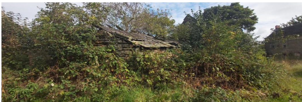
Fig 64 Former two-storey structure in state of collapse and overgrown
