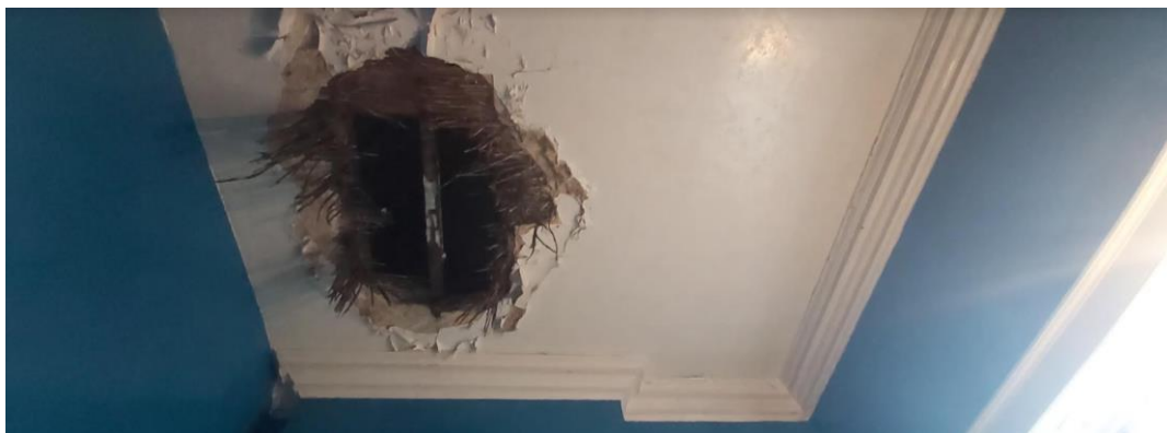
Fig 36 Water ingress has led to the collapse of a first floor, lath and plaster ceiling
