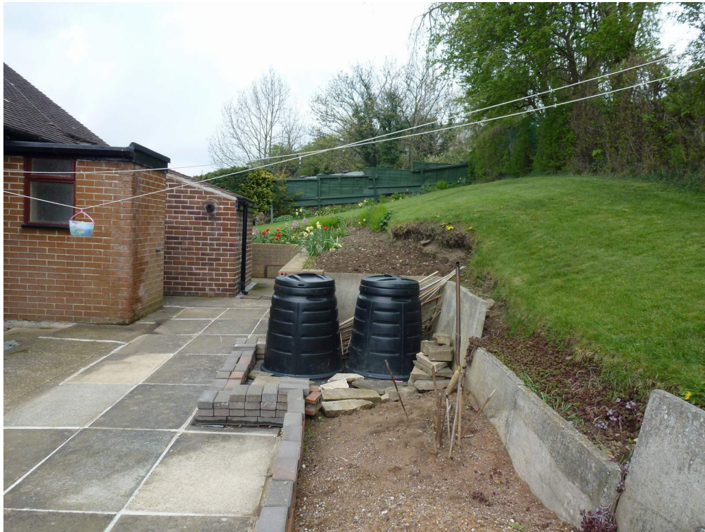
Photo 4 Rear garden area facing north showing existing retaining wall to garden. The edge of the lawn is the approximate line of the new retaining wall. The position of the car port will be towards the foreground of the photograph.
