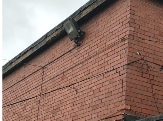
Image 20: Lifted felt on western side of Building 1
