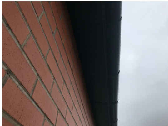
Image 22: Sealed fascias in Building 2
