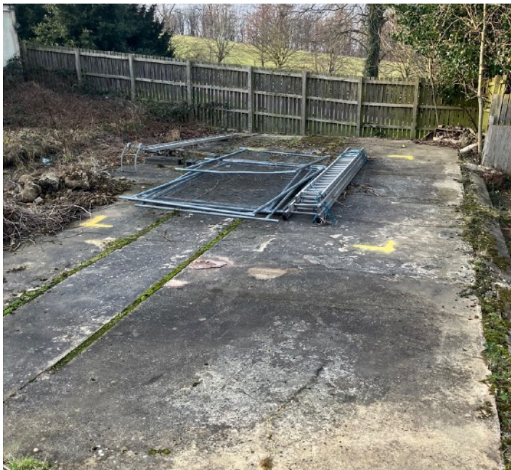
The existing hardstanding. The yellow lines indicate the proposed site of the greenhouse.
