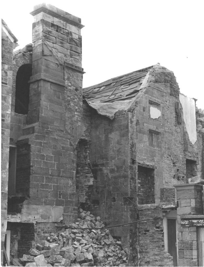
Photo of north elevation immediately following demolition indicating extent of repair works necessary.
