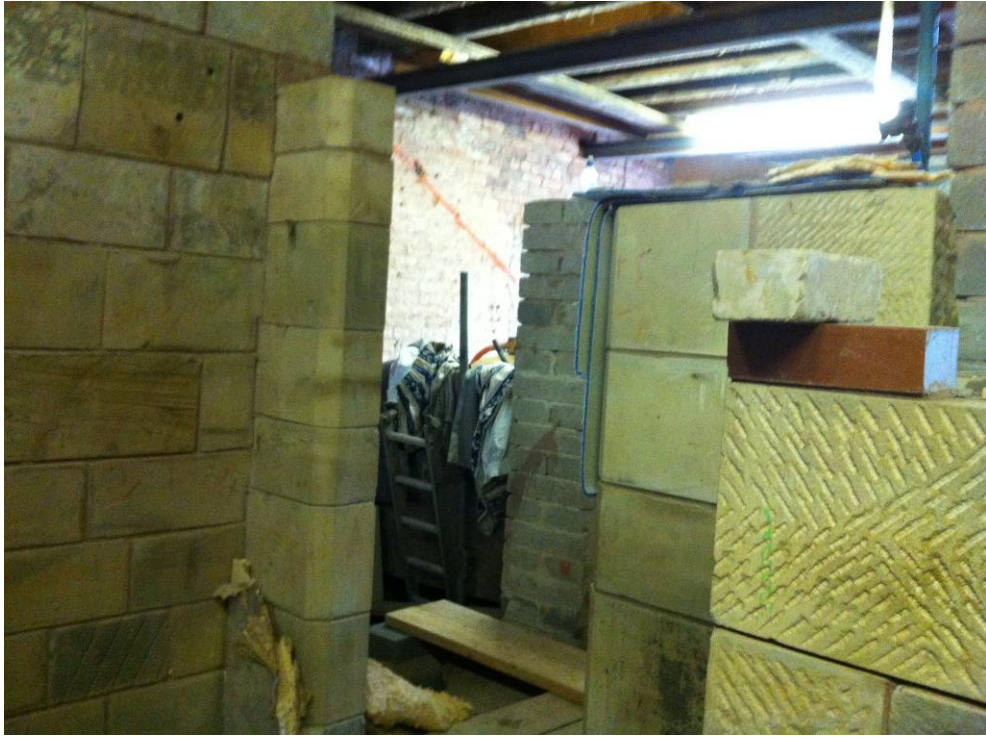
7. External view of new door opening D1 with corner of chimney stack in foreground.
