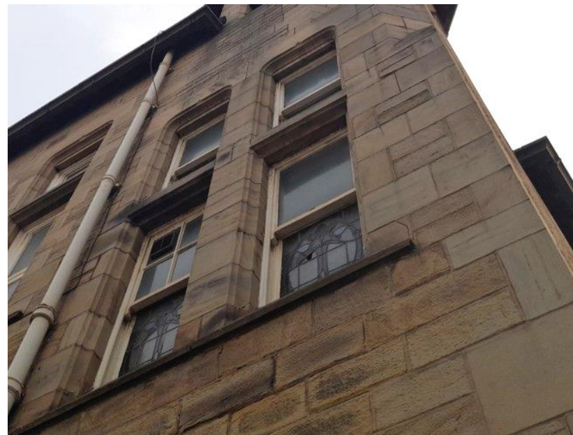
Figure 3 Missing glass in stained glass window.
