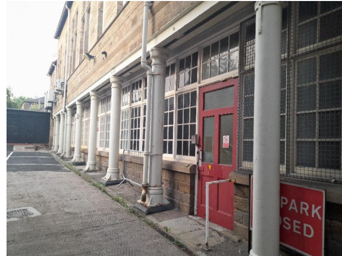
Figure 6 Colonnade; gaps between metal beams.
