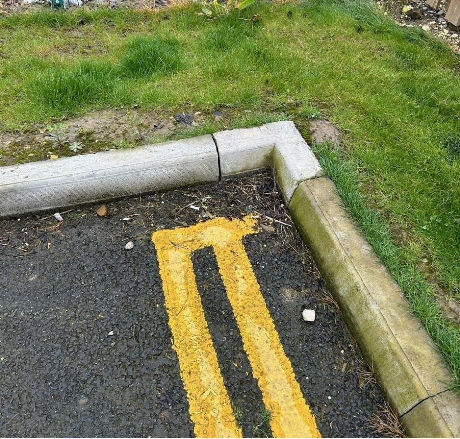
Image 12- Damage to corner kerb
