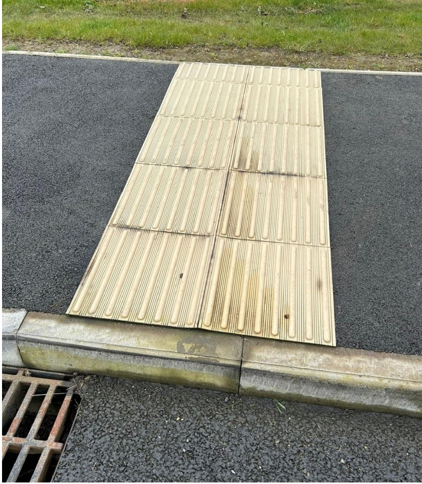
Image 7 – Corduroy warning surface lifting
