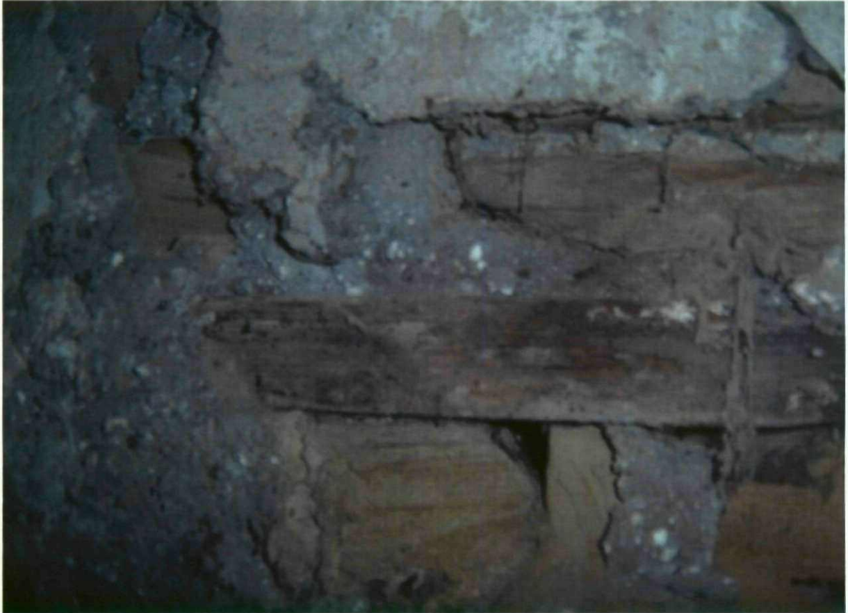
Timber Built into Wall
