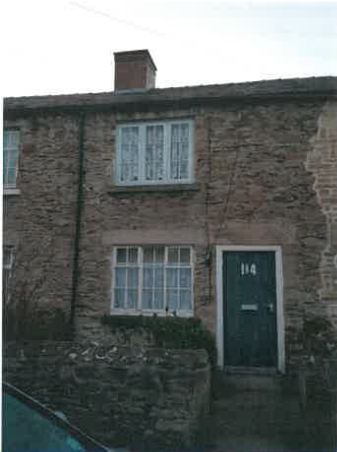
Figure 6 – Front elevation of the property – most of this area will require repair and repointing
