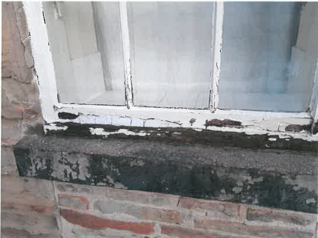
Figure 5 – Close up of existing ground floor rear window (left hand side) showing visible signs of decay
