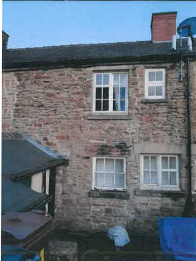
Figure 7 – Rear elevation of the property – most of this area will require repair and repointing. Just visible on the left hand side is the neighbouring property which has undergone similar works recently
