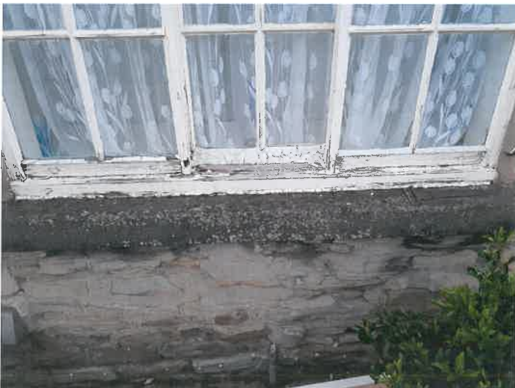
Figure 4 – Close up of existing ground floor front window showing visible signs of decay
