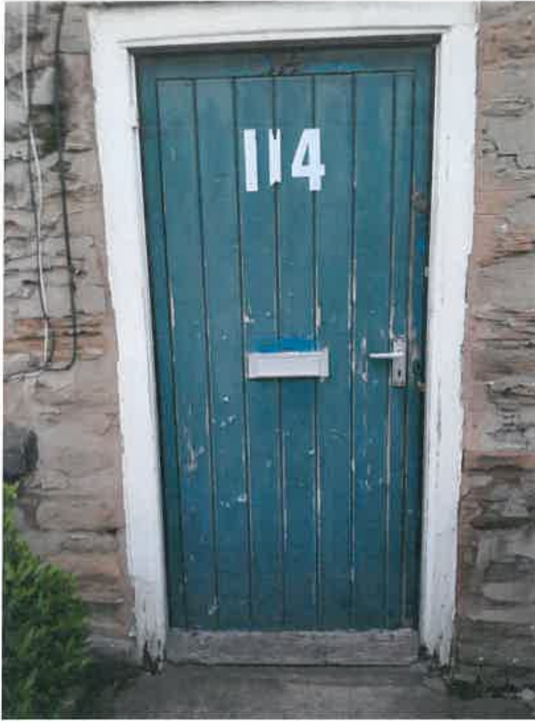
Figure 6 - Existing external front door with visible signs of decay
