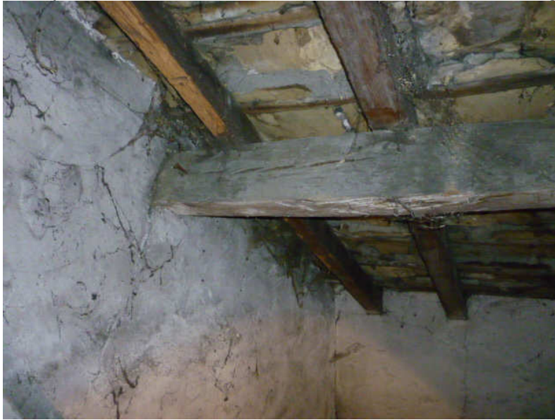
Photo 5: Showing level of webbing in roof timbers
