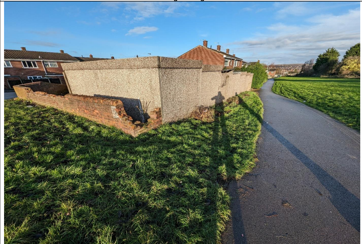
Photo 5 – View on rear of garages, on wall return, showing grass verge and path level
