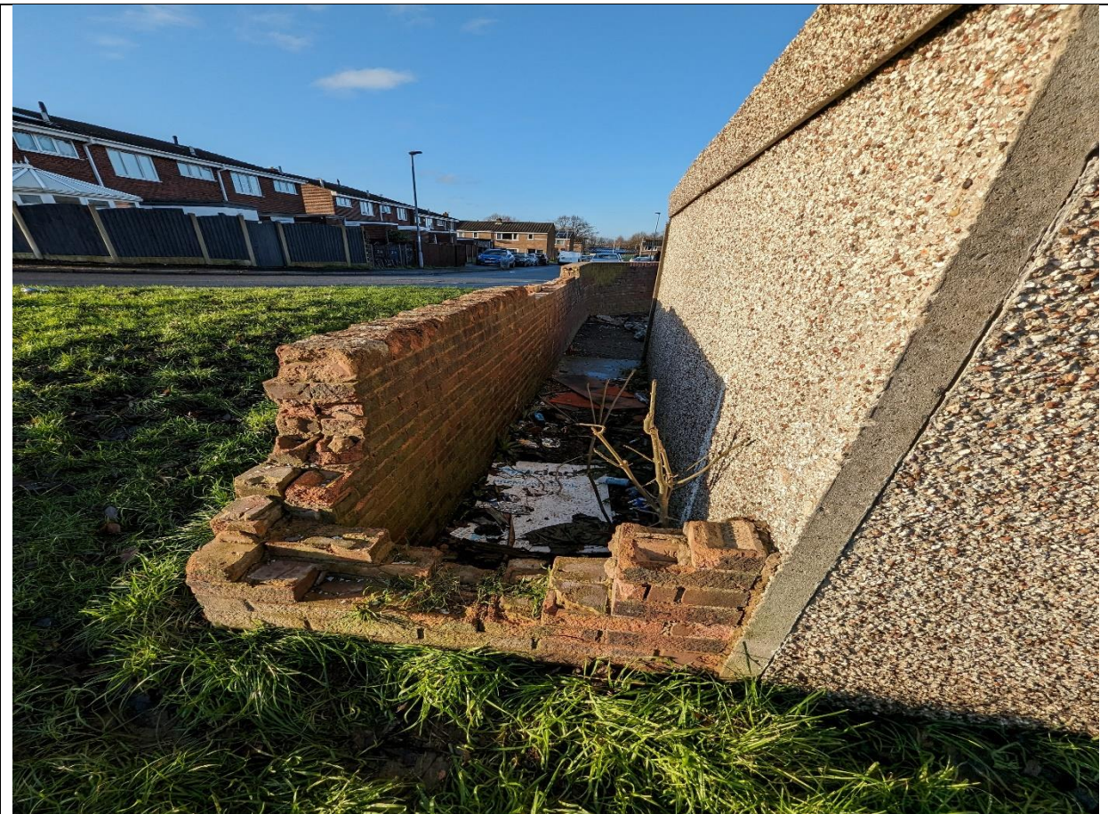
Photo 4 – View on return corner of wall showing damage
