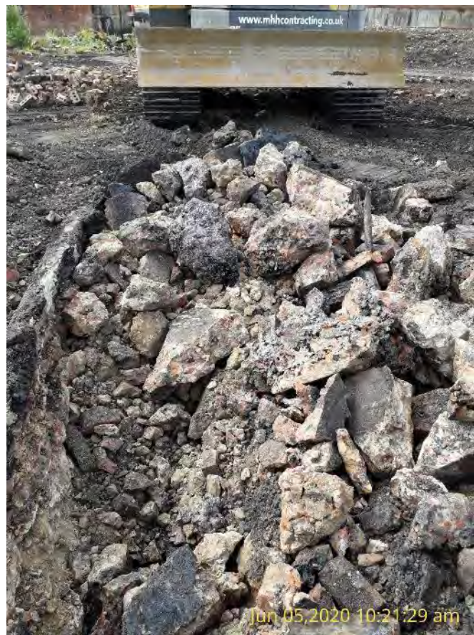
Photo 32: TP42 showing concrete obstructions
