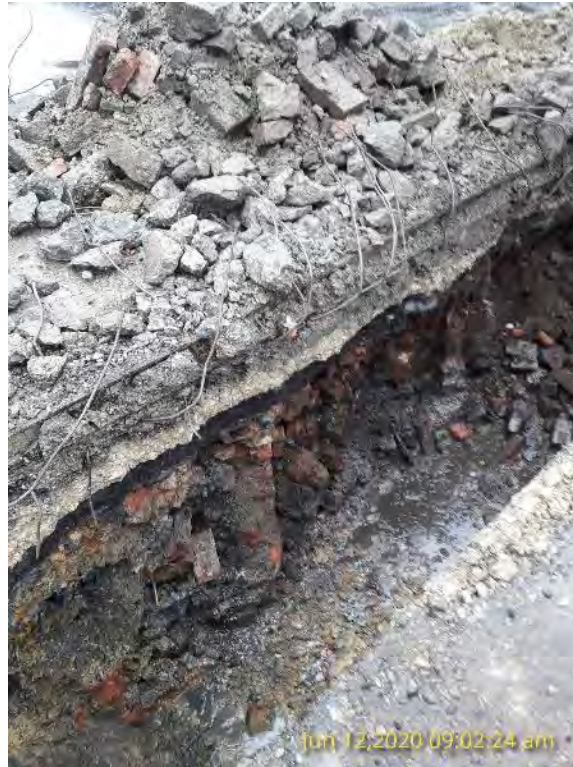
Photo 25: TP81 showing concrete and brick obstructions
