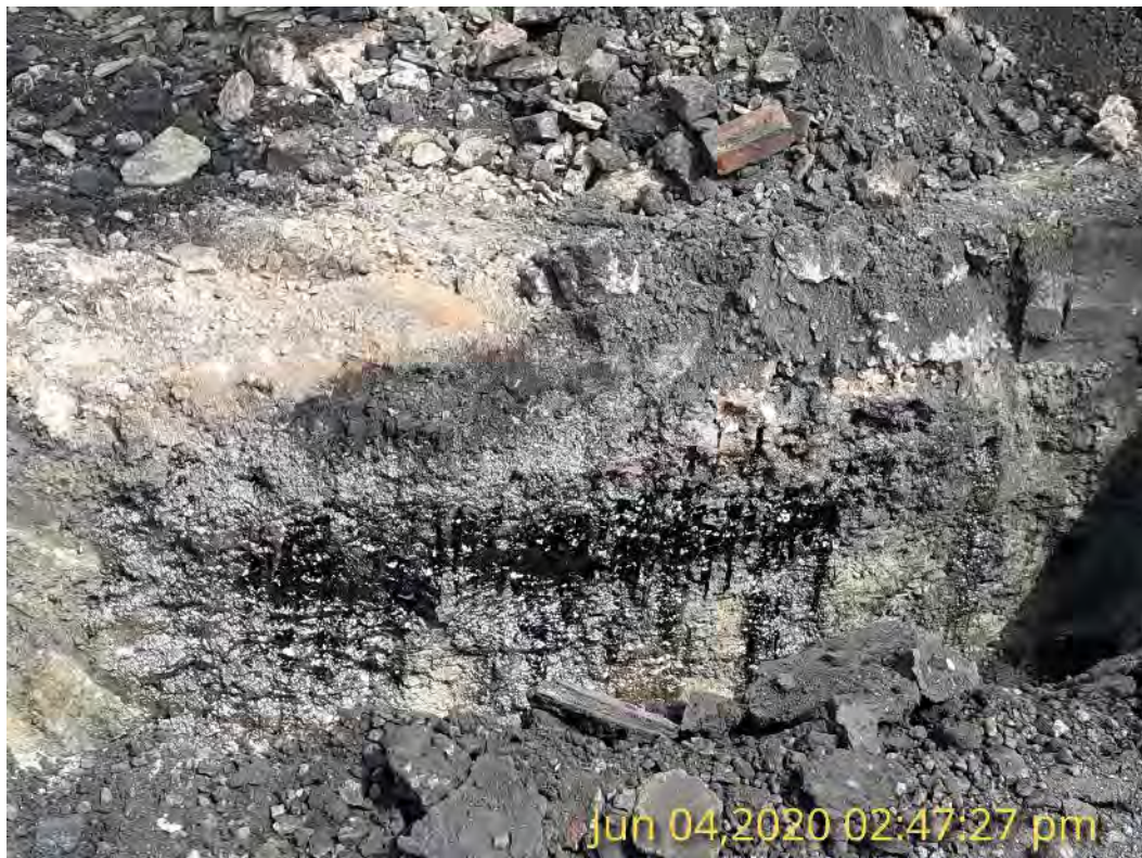
Photo 20: TP42 showing Coal tar seeping out of concrete
