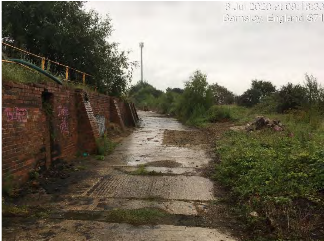
Photo 7: Retaining wall with evidence of coal tar staining located in the west of the Production Area
