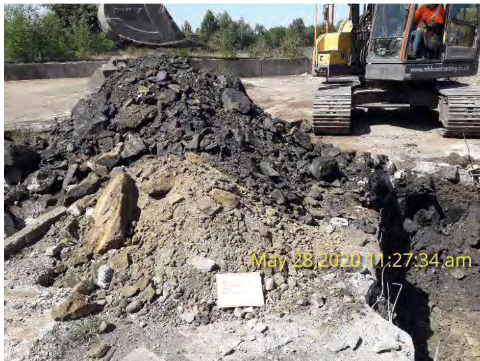
Photo 36: BH19-02 initial TP showing coal tar impact and infrastructure in pit.
