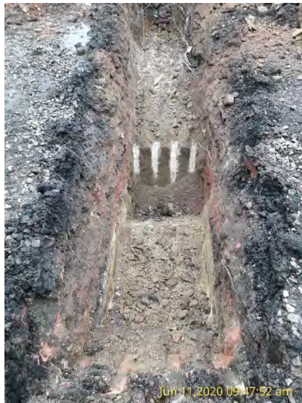
Photo 26: TP85 showing concrete obstruction.
