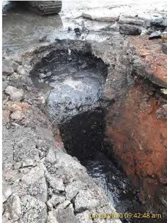
Photo 19: TP24 showing identified sump.
