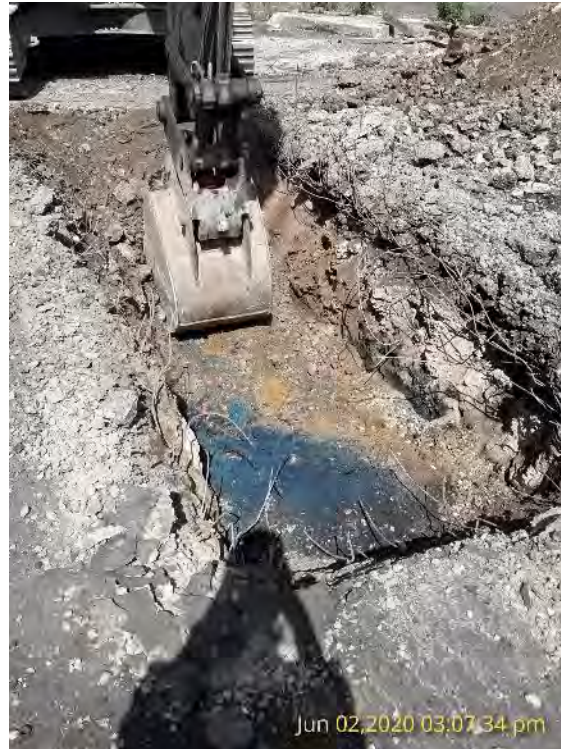
Photo 17: TP21 in Production Area showing blue stained soils (cyanide)
