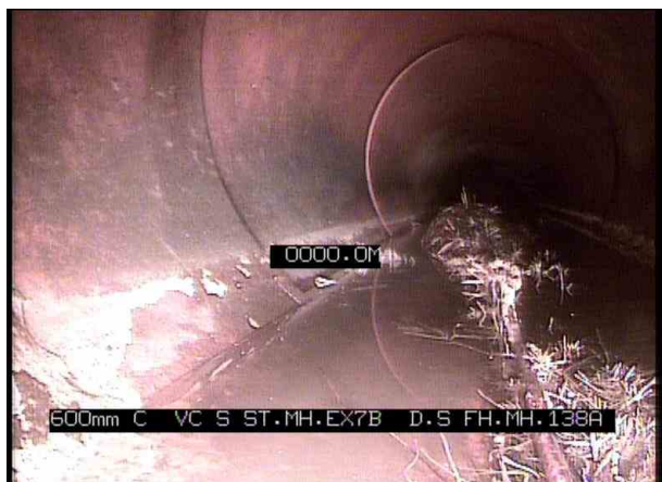
137BX_c6131b60-c190-4d2c-a1f4-2646fa072b78_20210923_113649_385.jpg, 00:00:00, 0.00 m Roots, mass, 10% cross-sectional area loss
