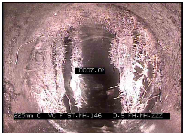
146X_250f062f-a501-4029-bb82-d4f1a554d51f_20210923_09 4515_705.jpg, 00:00:58, 7.00 m Roots, mass at joint, 20% cross-sectional area loss
