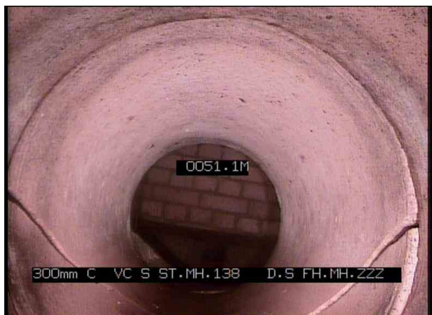
137X_a8ed3296-1cac-4ba0-9d41-4840c77ce783_20210921_105322_318.jpg, 00:05:09, 51.10 m Fracture, circumferential at joint from 3 o'clock to 9 o'clock
