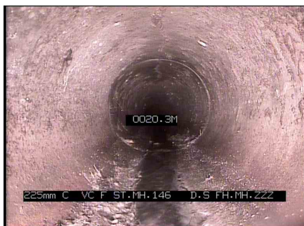
146X_81b8881c-ab65-40b9-a9f1-5c5a30919911_20210923_0 94713_906.jpg, 00:02:43, 20.30 m Fracture, longitudinal at 6 o'clock
