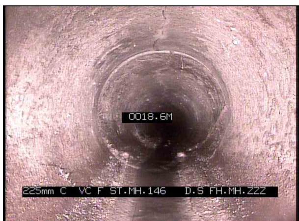
146X_e4c12ad6-a9f6-4cfe-8253-43950971168f_20210923_09 4645_410.jpg, 00:02:19, 18.60 m Fracture, longitudinal at 12 o'clock
