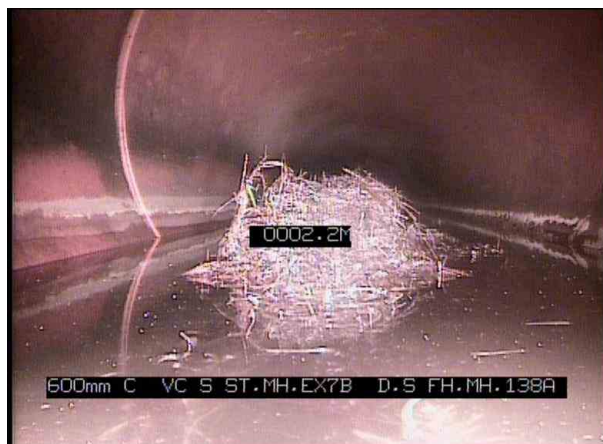
137BX_c5f92405-0081-4295-9ede-4fb2628d24ff_20210923_113910_768.jpg, 00:01:35, 2.20 m Roots, mass, 20% cross-sectional area loss
