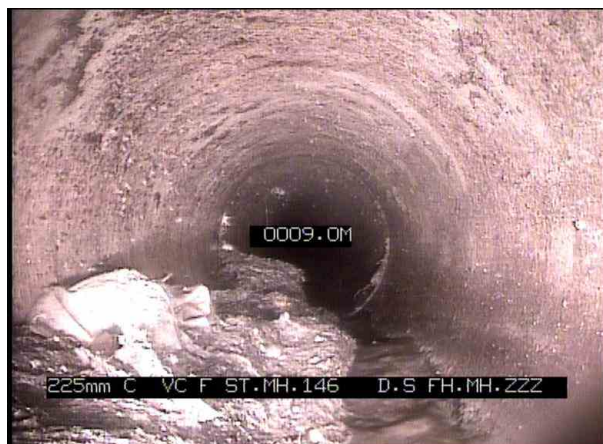
146X_b49e6835-9183-42c0-89ac-85fd8a292636_20210923_0 94543_089.jpg, 00:01:21, 9.00 m Roots, mass, 25% cross-sectional area loss
