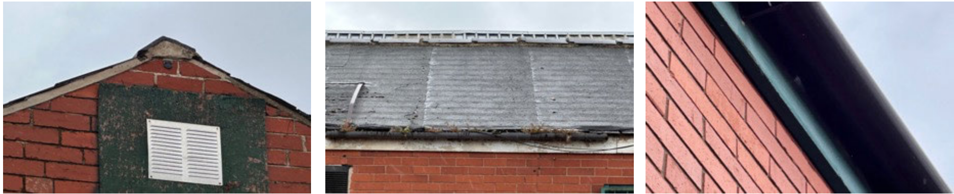
Images 7-9: North elevation of B1 (left) – north elevation roof structure with bitumen style lining (centre) – example of the intact barge boards (right)
