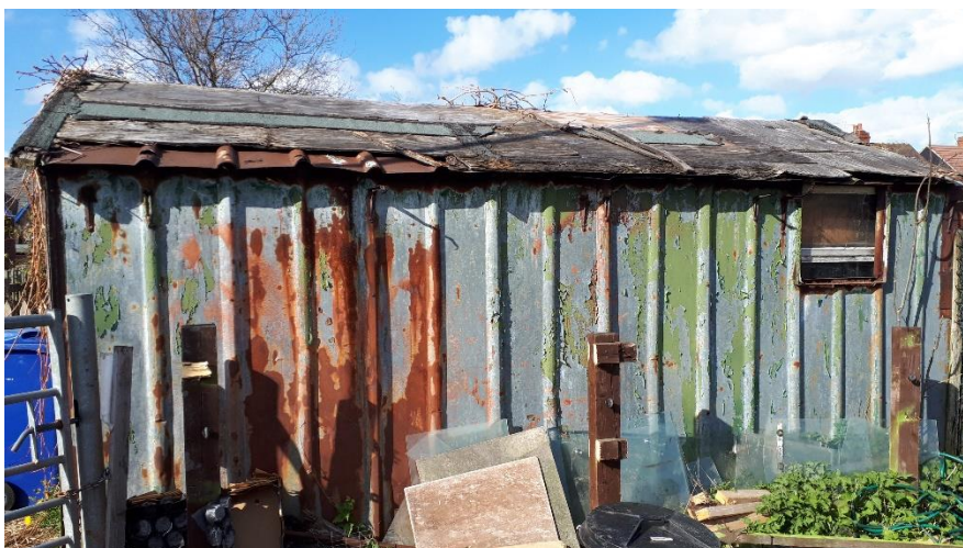
Photograph 1: Building B1 with gappy composite roof.
