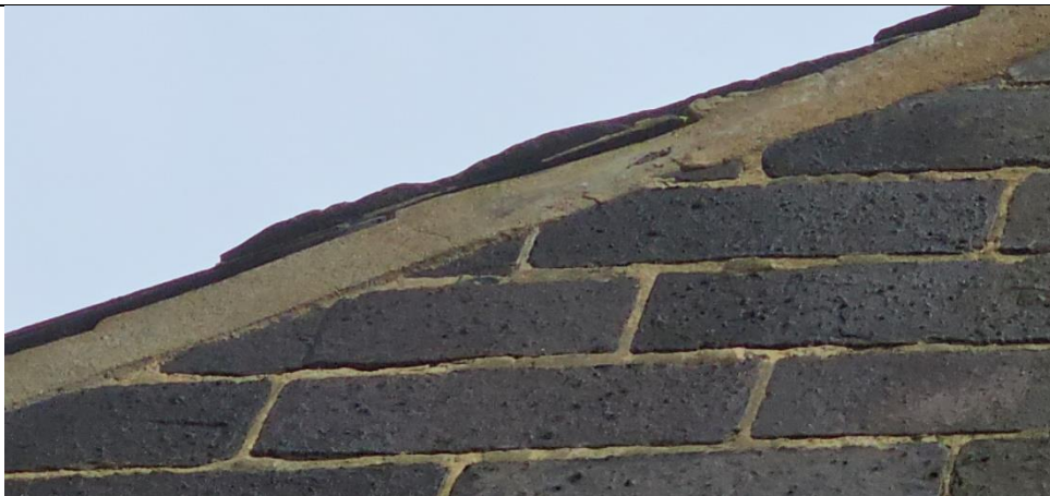
Photo 5 gap along the verge of the gable.
