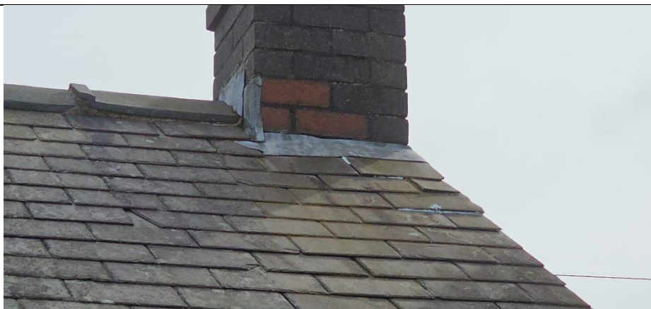
Photo 8 left tiles and gap under ridge tile.
