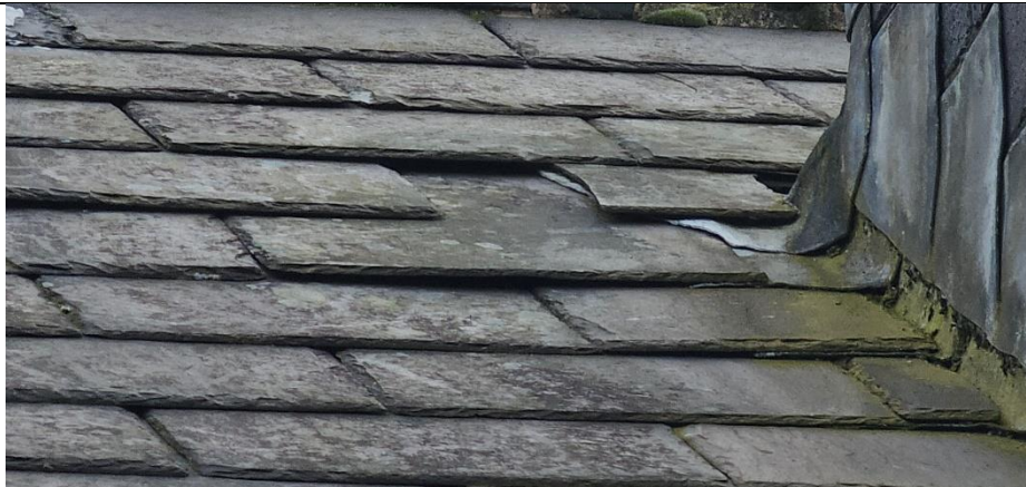
Photo 7 Shifted tiles/broken tiles near the chimney.
