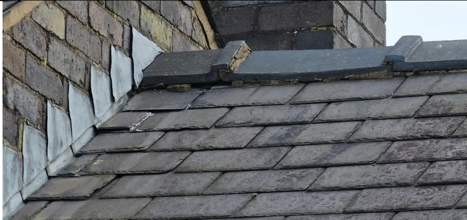
Photo 6: missing mortar and a gap under the ridge tile.
