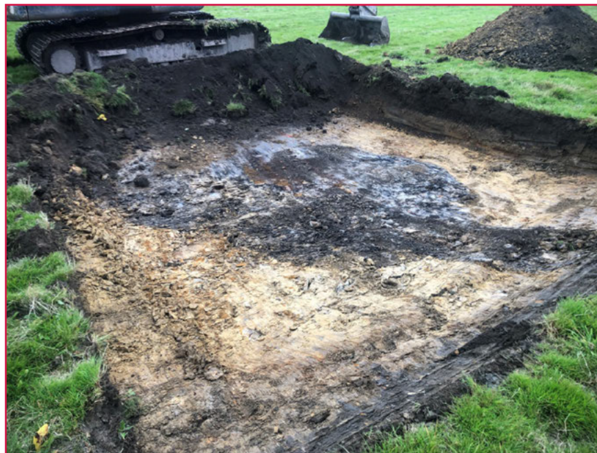
Figure 6 – Encountered Mine Shaft
