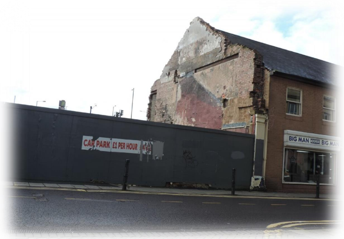
Fig.8: Photo showing the site from Wellington Street, opposite 2no Grade II listed buildings. The temporary hoarding and damaged gable end substantially detract from the character of the area and undermine the setting of the listed buildings.
