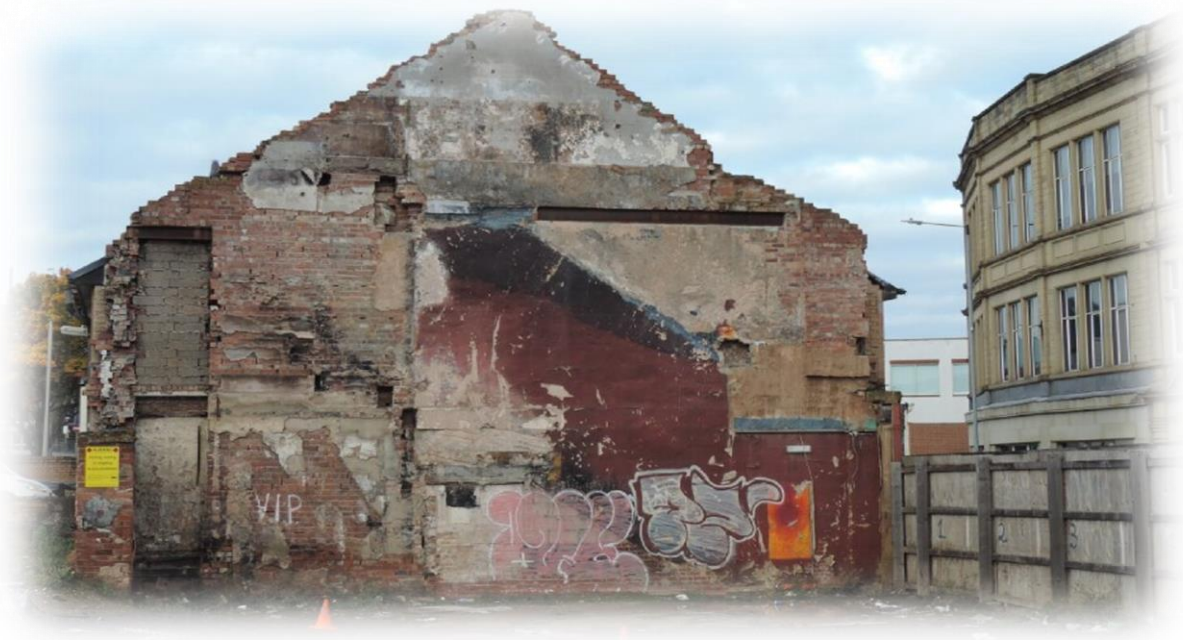
Fig.7: Photo showing the existing exposed, damaged and graffitied gable end which can be seen from west way, New Street and Wellington Street.
