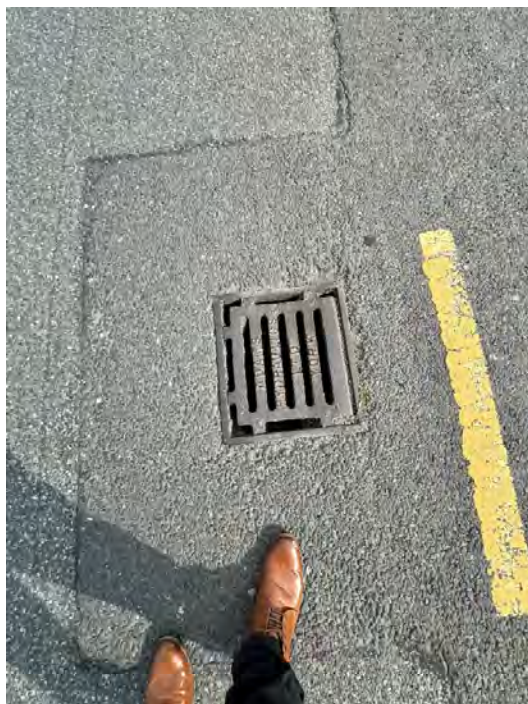
35 -Close up of gully ,
