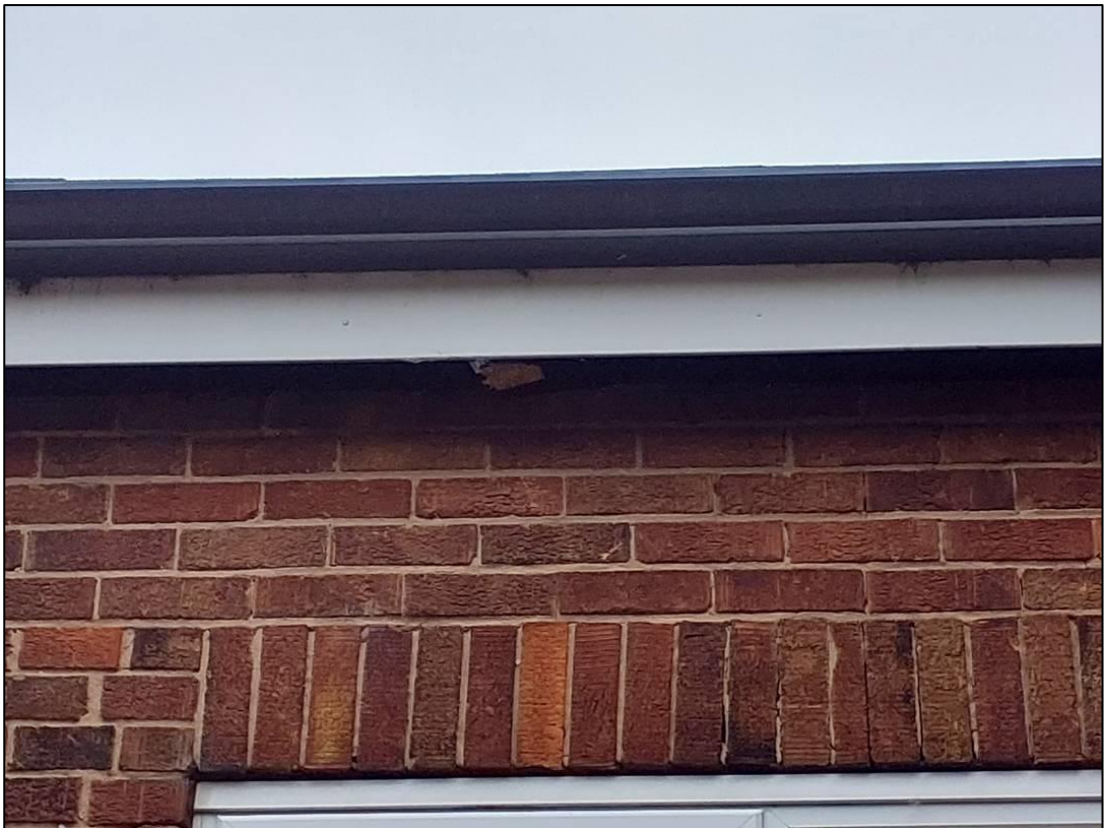
Photograph 9: Gap in soffit on B1
