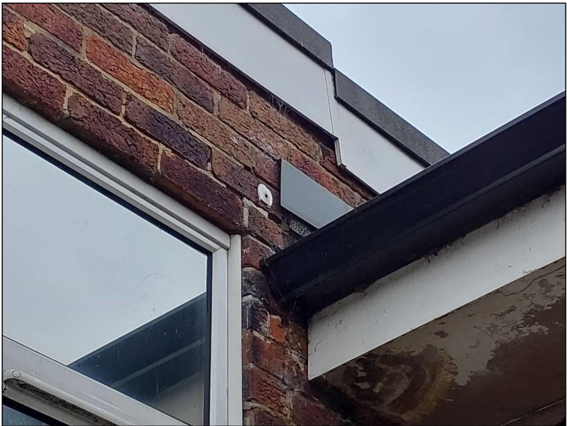
Photograph 10: Gaps under soffit on B1
