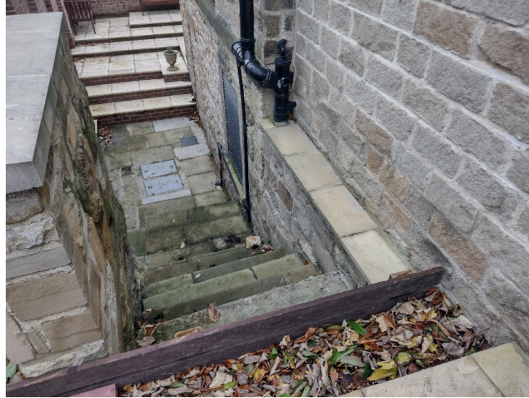
Fig 19: Existing steps between boundary and north-west wing – uneven length, height and width.
