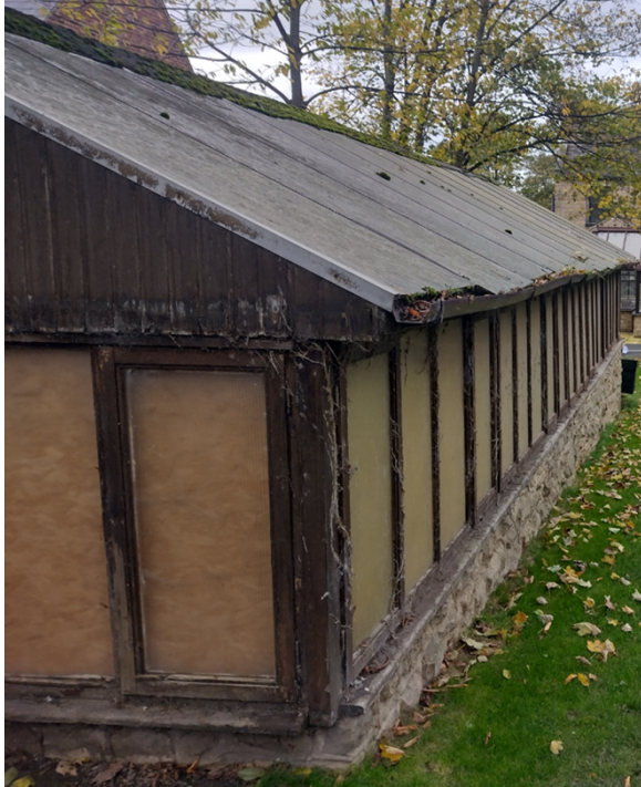
Fig 10: Slipped roof panels, and rotten corner post
