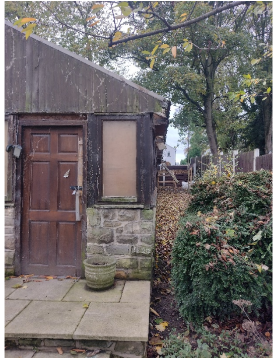
Fig 11: Inappropriate door and poor verge detail
