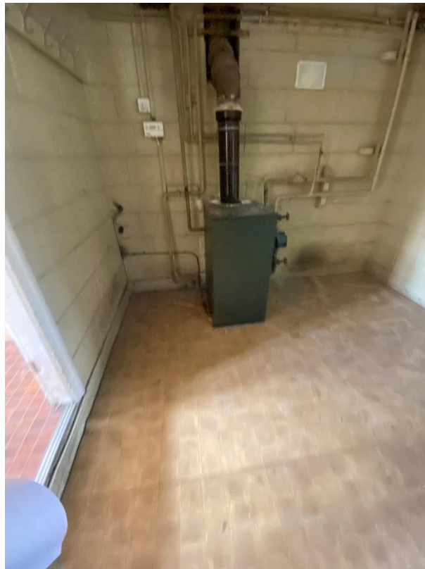
Figure 34 Boiler in lobby/boot room.
