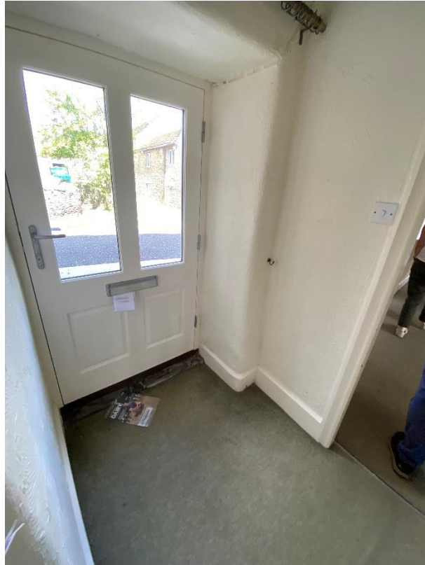
Figure 40 Entrance lobby Historically this was a window and the lobby has been partitioned in.
