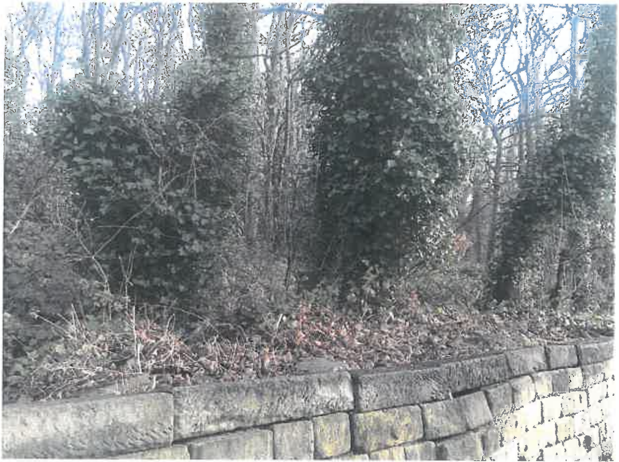
Photo 3 – View from No 87 Showing Bulging, Misalignment to wall, and close Proximity of Trees to the Wall
