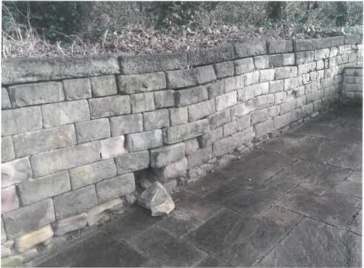
Photo 2 – View from No 87 Showing Bulging, Misalignment to wall and Masonry Dislodging from Wall
