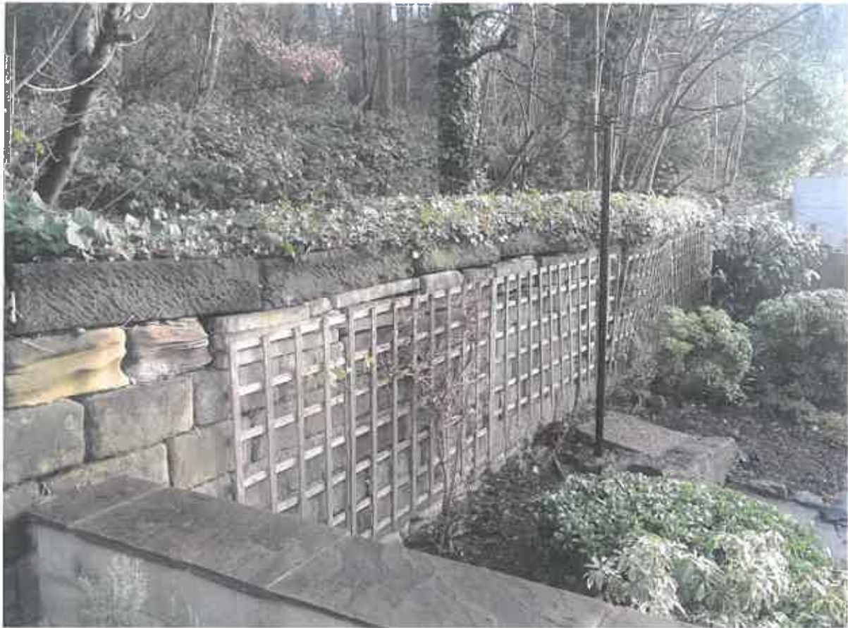
Photo 4 – Right Hand Side View from No 87 towards No 89 Showing Bulging, Misalignment to wall, and close Proximity of Trees to the Wall
