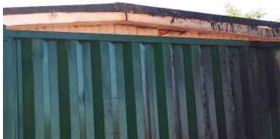
Photograph 3: B4 (damage to northern gable)
