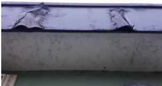
Photograph 5: B3 (delaminating fascia)
