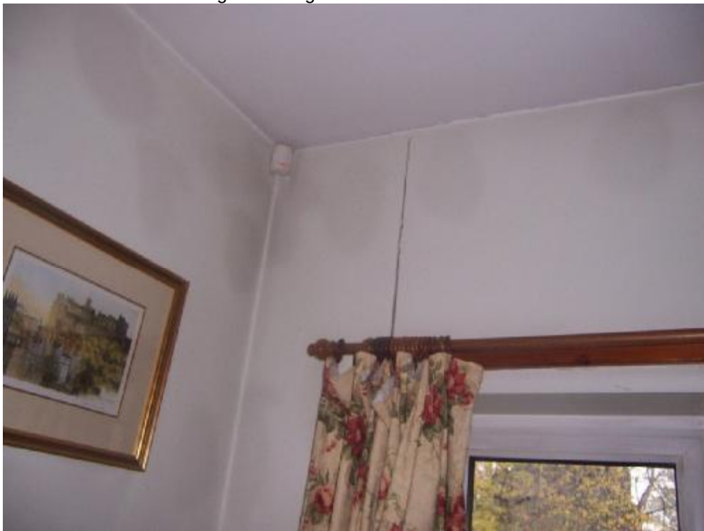
FIGURE 4 Internal damage to lounge
