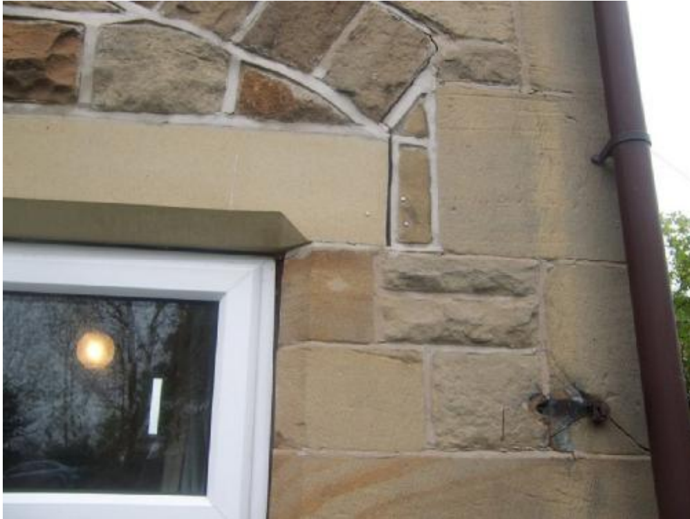
FIGURE 3 External damage to cottage
