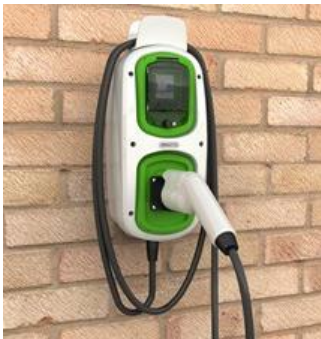
Typical example of a wall mounted electric vehicle charging point
