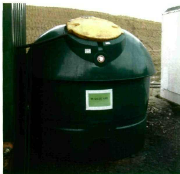
Waste oil storage
