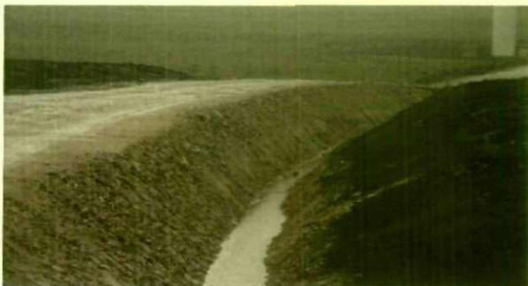
An example of drainage alongside tracks
