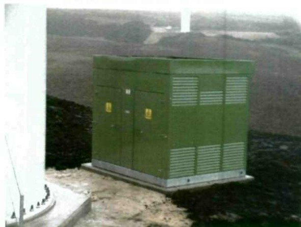
A bunded transformer
