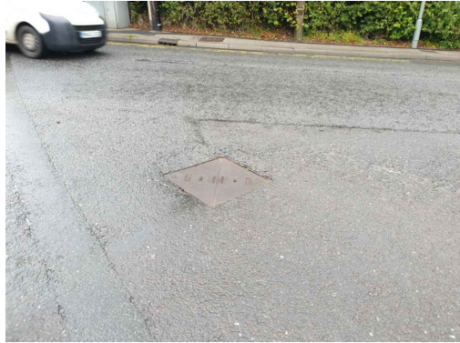
4 - Scarring on tarmac and footway. Manhole sunk. Kerb and gully misaligned
