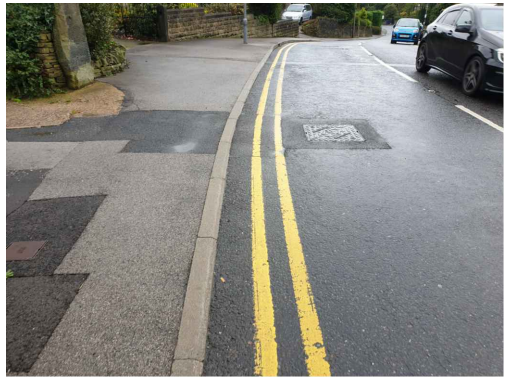
7 - Scarring and fretting on footway and highway. Kerbs damaged and misaligned. Footway damaged by driveways to the left
