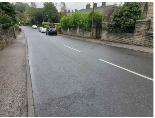
9 - Scarring and fretting on footway and highway. Kerbs damaged and misaligned.
