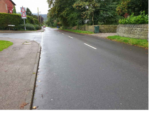
14 - Scarring and fretting on footway. Kerbs damaged and misaligned. Footway tarmac cracking and damaged
