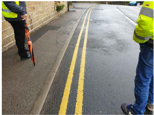
6 - Scarring and fretting on footway and highway. Kerbs damaged and misaligned
