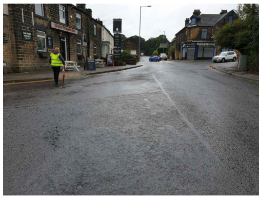
3 - Scarring on tarmac and footway. YW vales and manhole sunk
