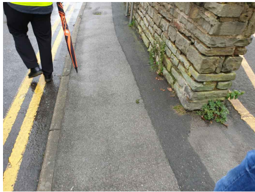
5 - Scarring on footway. Kerbs damaged and misaligned
