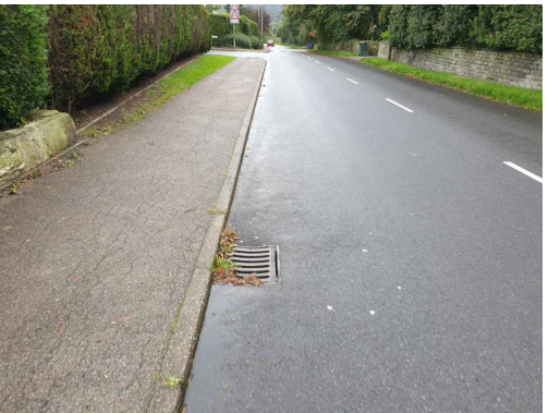
12 - Scarring and fretting on footway. Kerbs damaged and misaligned. Footway tarmac cracking and damaged
