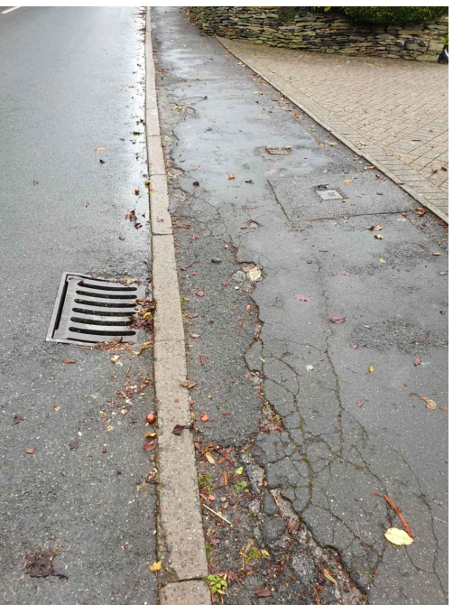
16 - Footway badly damaged with wearing course coming away. Kerbs damaged and misaligned.
