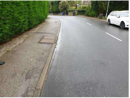
10 - Scarring and fretting on footway and highway. Kerbs damaged and misaligned. Footway tarmac cracking and damaged
