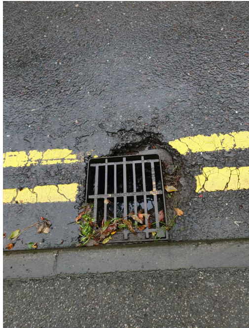
2 - Tarmac damaged around gully
