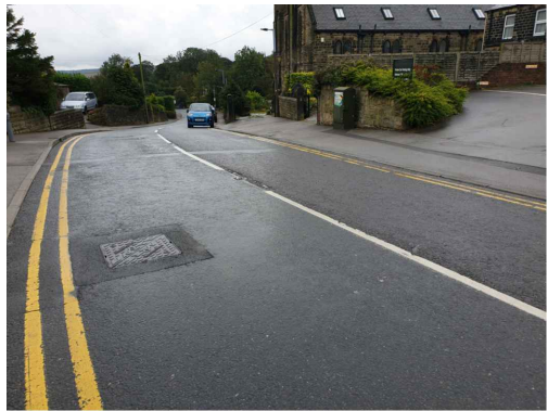
8 - Scarring and fretting on footway and highway. Kerbs damaged and misaligned. Fretting around manhole patch
