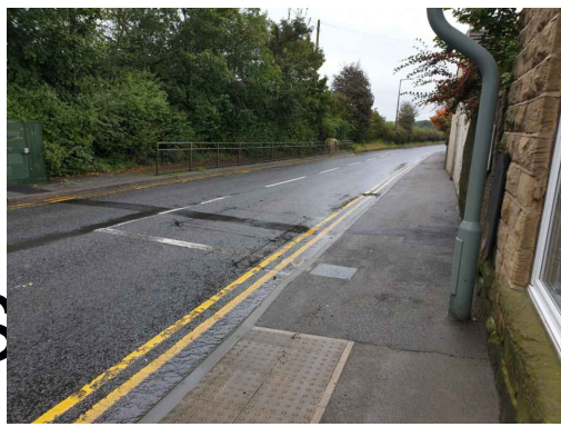
1 - Scarring on highway and footway, kerb damage.
