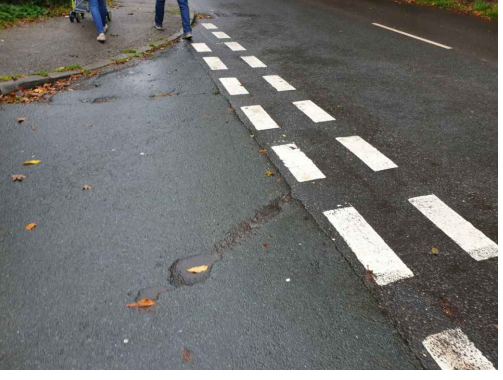
15 - Tarmac on highway damaged. Joint on junction is fretting. Kerbs damaged and misaligned. Footway tarmac cracking and damaged
