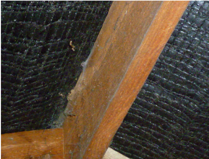
Photo 2: Webs on roof timbers
