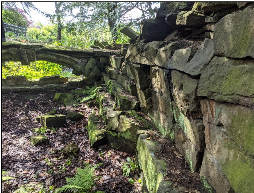
Photo of part of the plunge pool with loose stones in foreground and the crossing bridge in background
