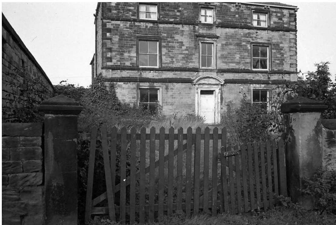
fig. 4 - 1980s photograph showing the property significantly dilapidated.
