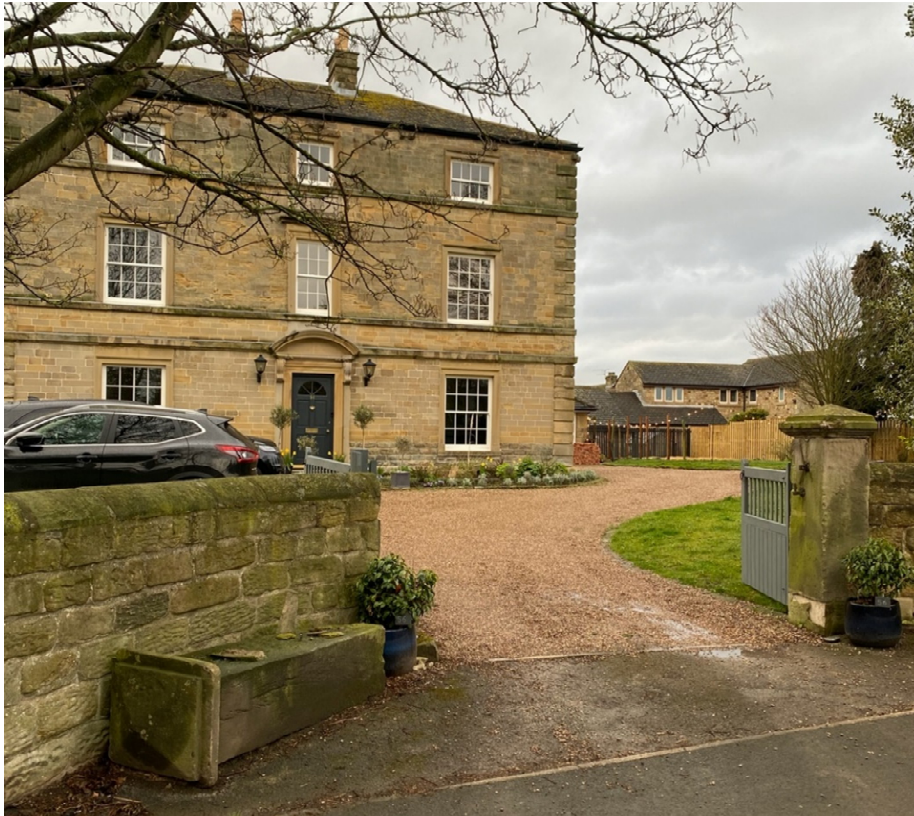
fig. 11 – Gate pillar knocked over by a previous owner will be reinstated with these newly proposed works
