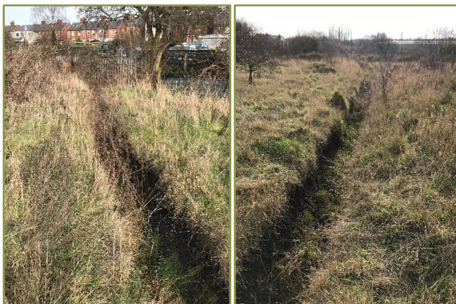
Left: View north along Drainage Cut. Right: View south along Drainage Cut.
