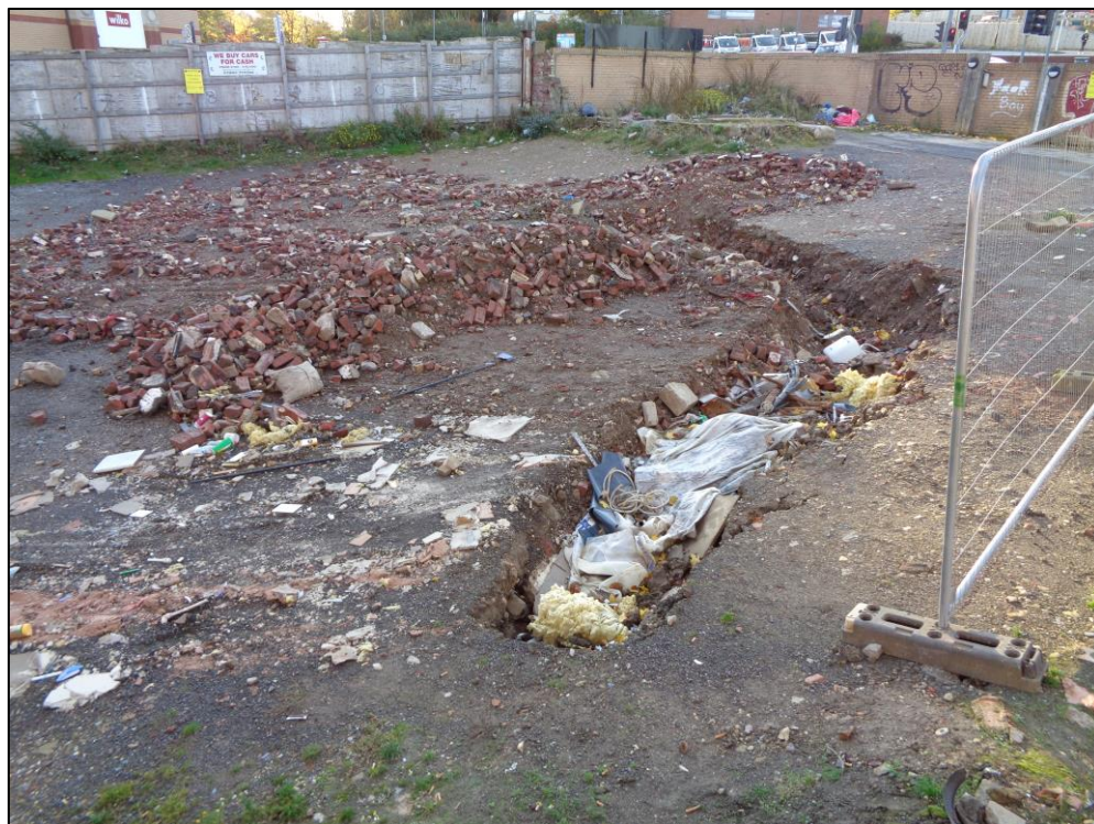
Plate 4: View looking SW showing trench dug within area of hardstanding towards the SW corner of site
