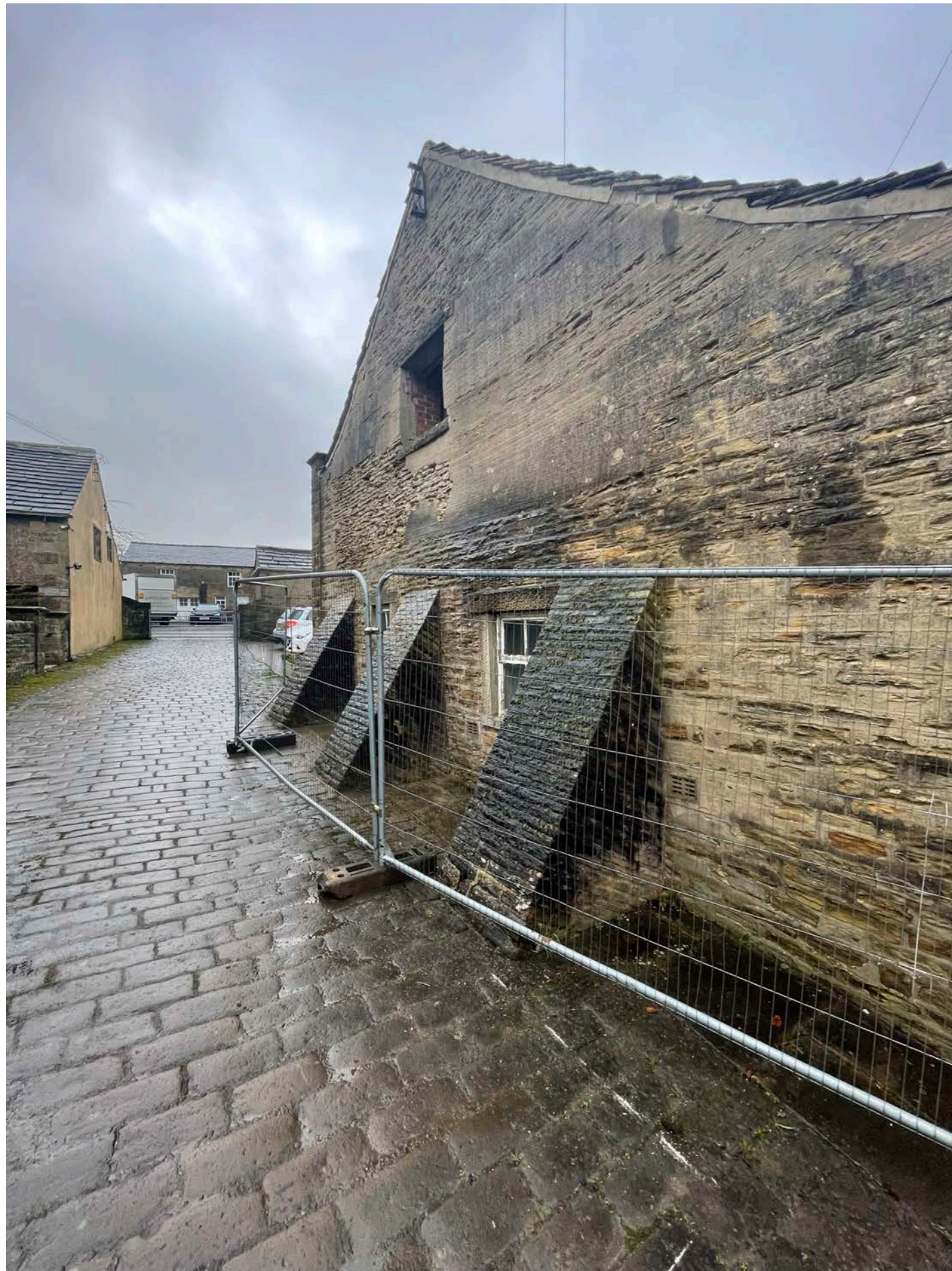
View of the existing gable with render partially removed, Evidence of 'bowing' wall pushing out above the buttresses
