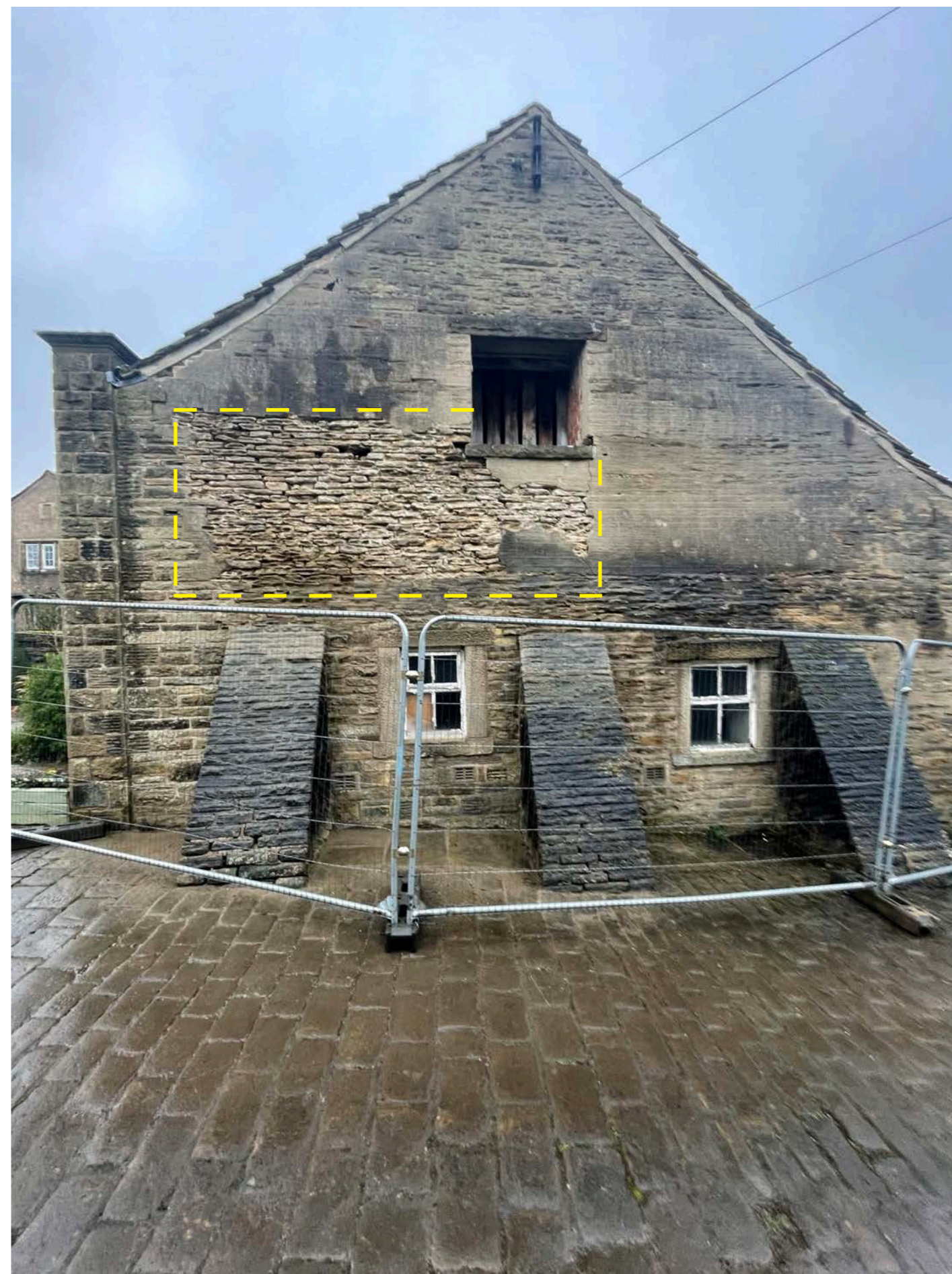
View of the existing gable with render partially removed, Evidence of loose stonework is identified by the yellow dotted lines
