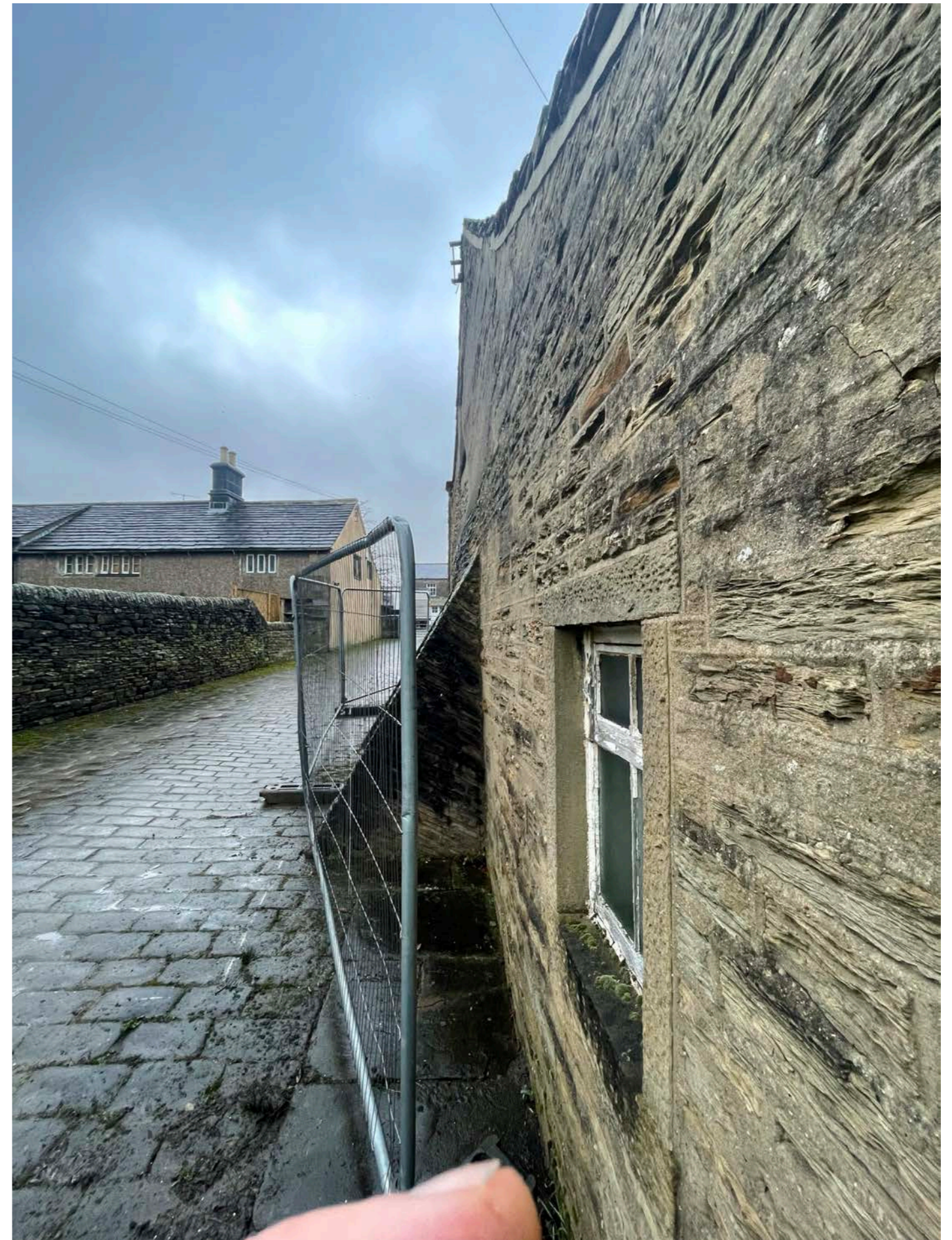
View of the existing gable with render partially removed, Evidence of 'bowing' wall pushing out above the buttresses
