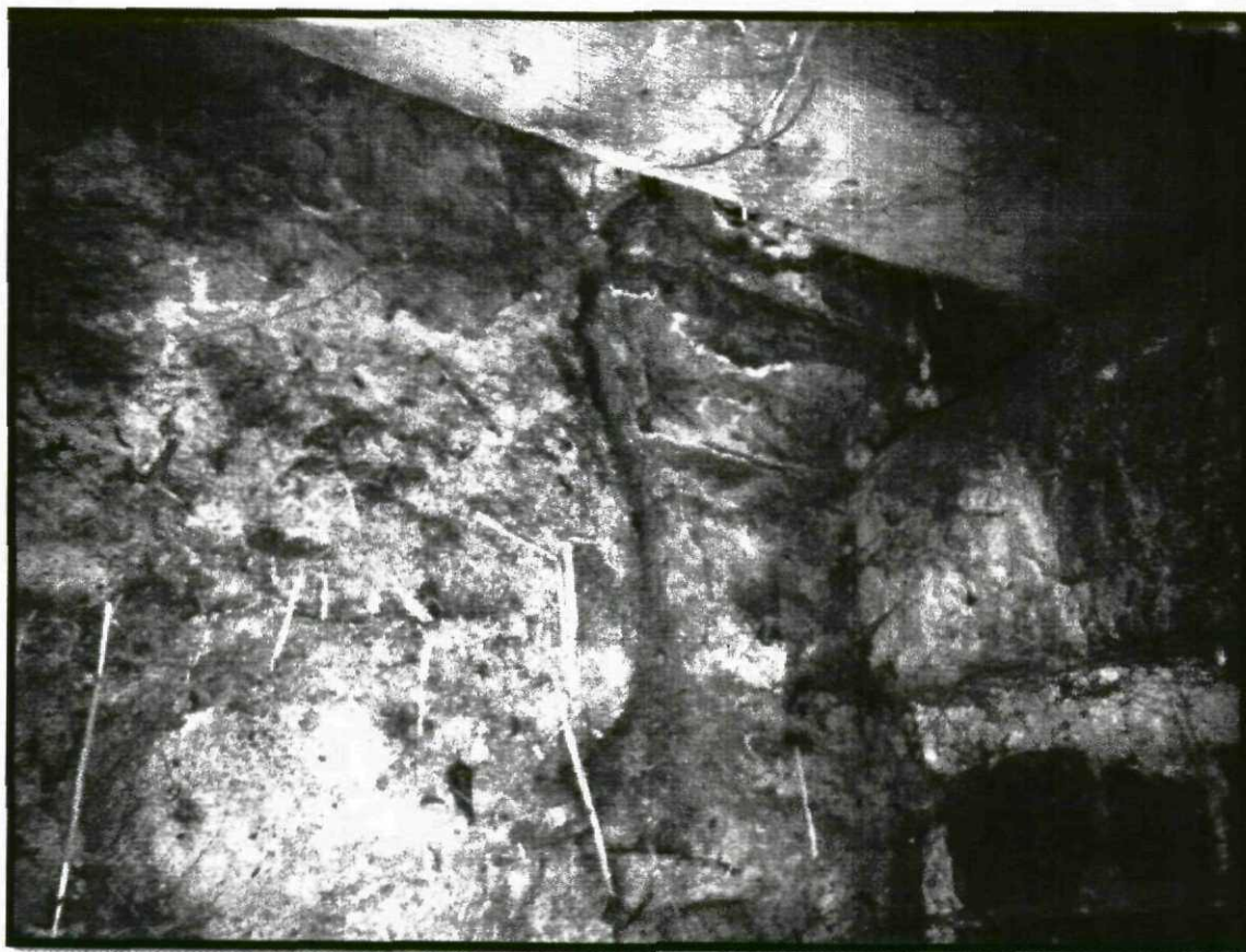
Photograph 69 – View of crack to window in North Elevation
