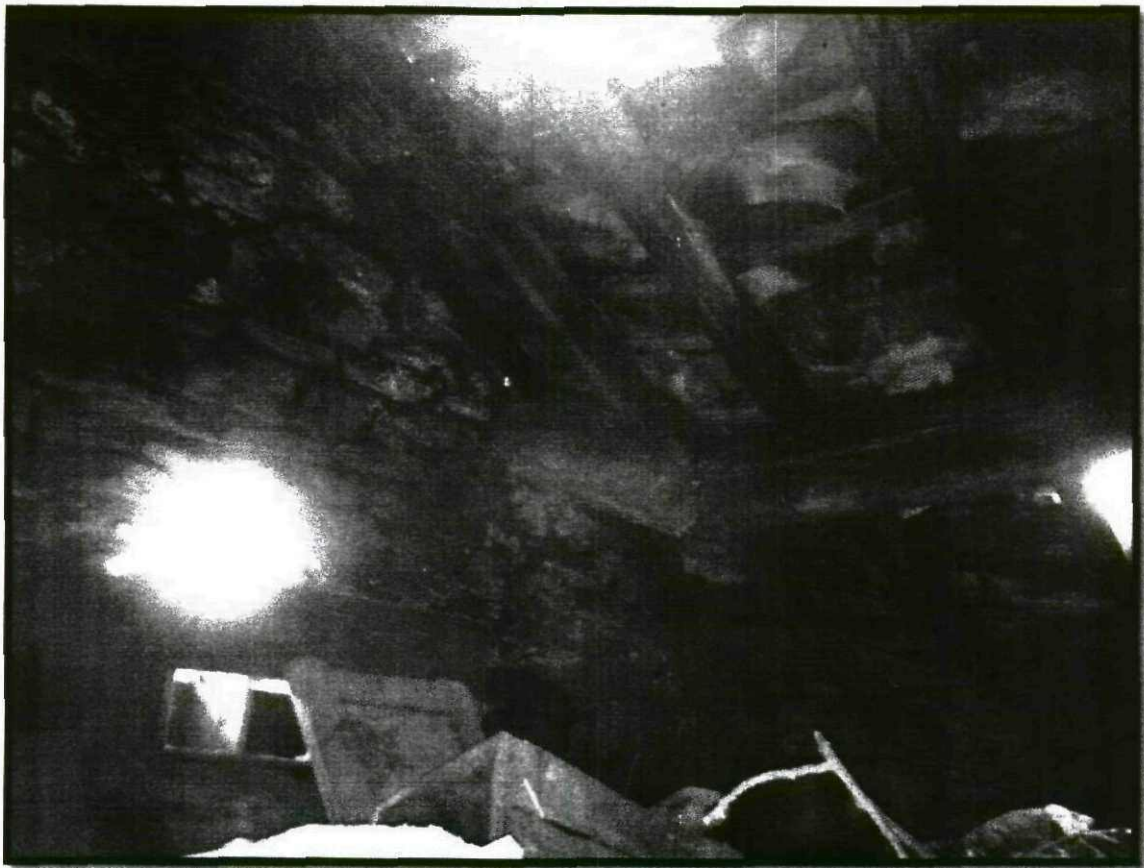
Photograph 59 – View of failed purlin
