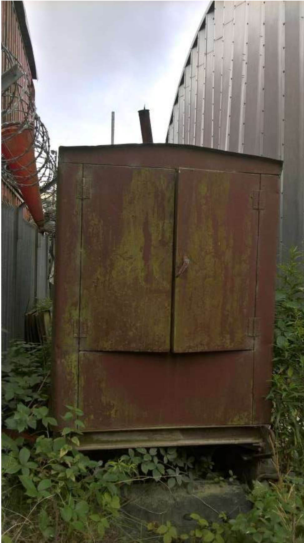
4. Diesel electricity generator located to the south of the on-site structure.
