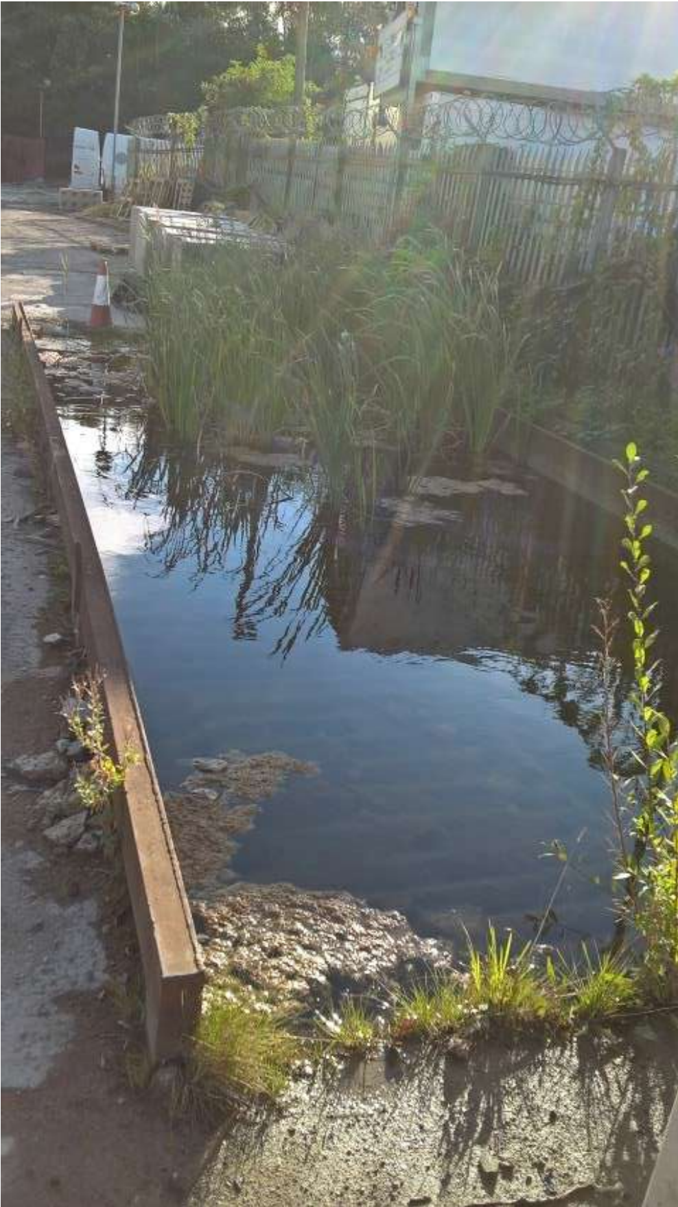
26. Weighbridge pit filled with essentially clear rainwater. Located west of north-west corner of the site of interest, along the access road into the site of interest.
