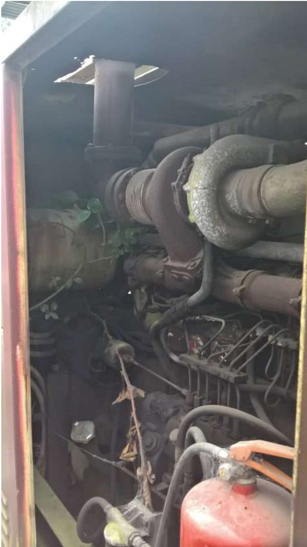
5. View inside disused diesel generator.
