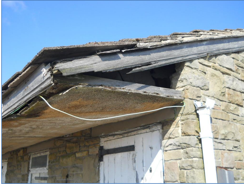
Figure 3: B1 Gap in soffit box, overhanging tiles, and missing mortar southeast corner.
