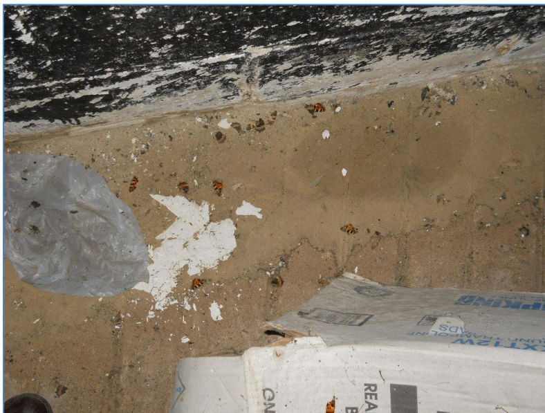
Figure 6: B1 prey remains located below gaps in wall tops on northwestern internal wall.
