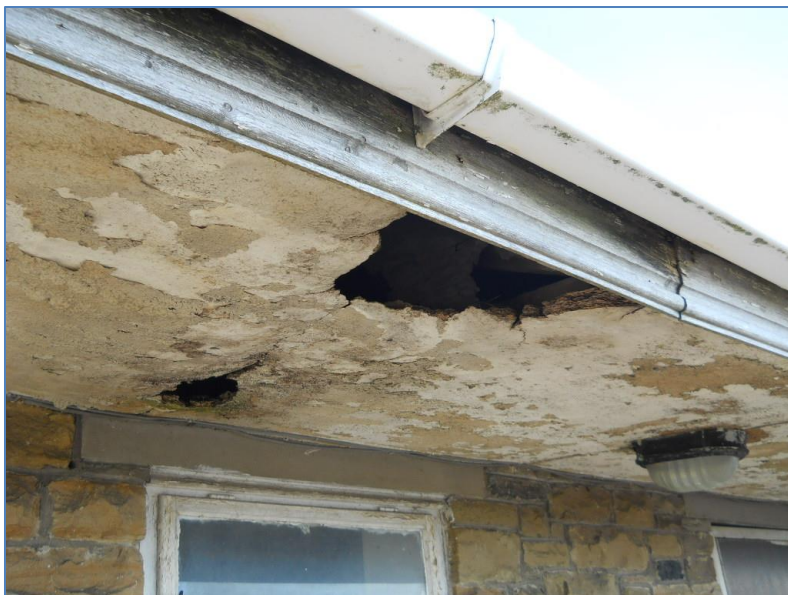
Figure 2: B1 holes in large wooden soffit box southwest elevation.
