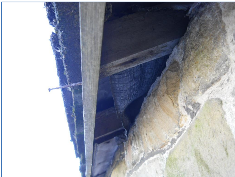
Figure 4: B1 northeast elevation missing boards on underside of wooden soffit box with exposed wall tops and roofing felt visible.
