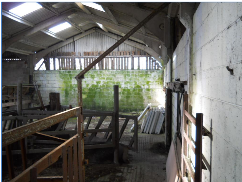
Figure 12: Building 3 (B3) interior – missing wooden planks on northwest elevation.
