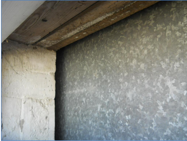
Figure 5: B1 window on northeast elevation boarded internally with gaps visible.
