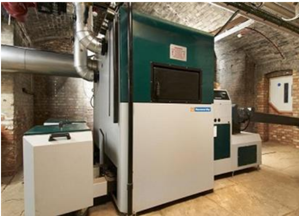
Figure 15. Commercial biomass boiler 6
