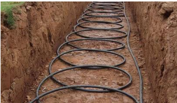
Figure 13. Horizontal ground loop collector 4
