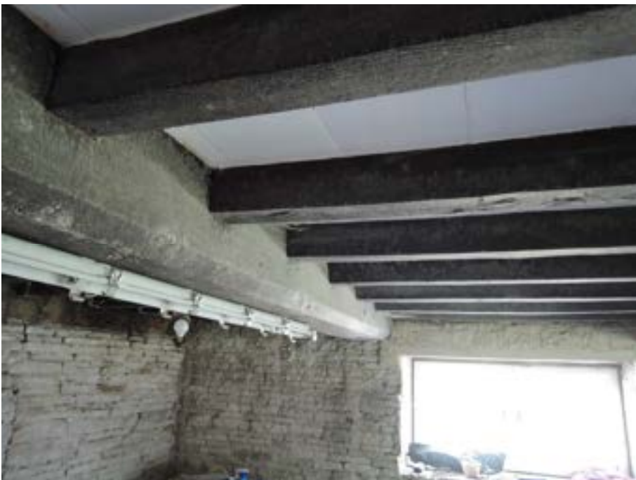
Dining room ceiling. First floor joists and beams in good order (subject to specialist inspection for rot/insect attack). Acceptable bounce under drop heel test.
