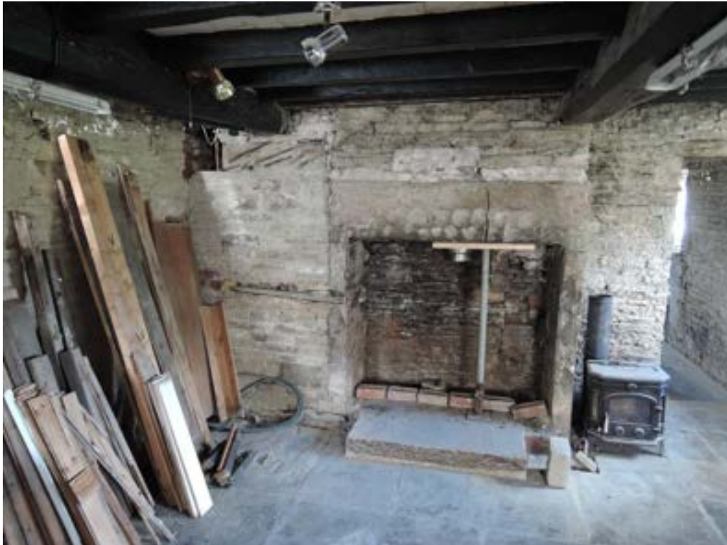
Living room fireplace. Cracked mantel stone with acrow prop. Right cheek wall has yielded out to the right following bending failure of mantel.
