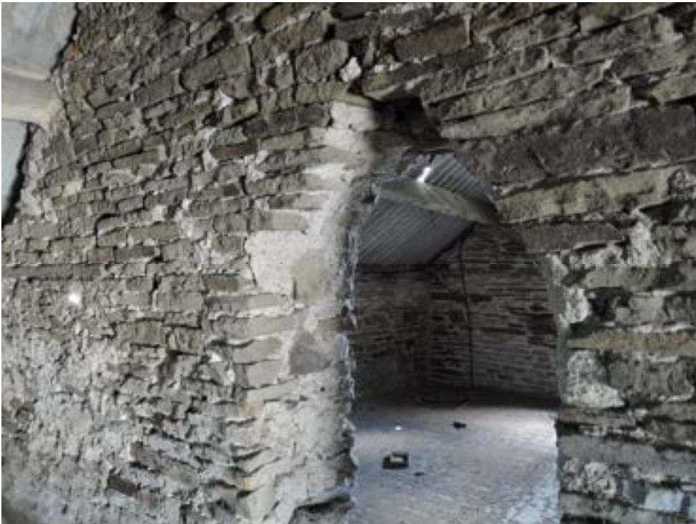
Inner wall first floor. Light repair required at head of arch
