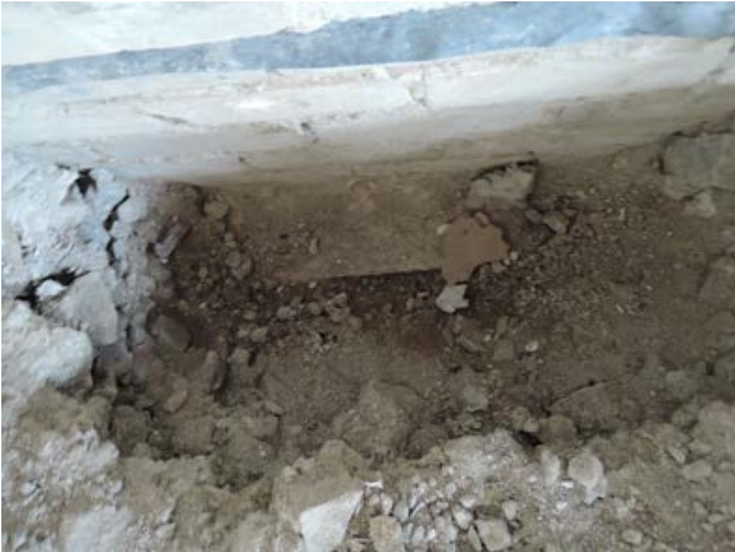
Trial pit showing foundation as concrete with 150mm projection at 300mm below slab. Foundation approx. 500mm – 600mm wide overall and therefore has capacity to support another proposed storey.
