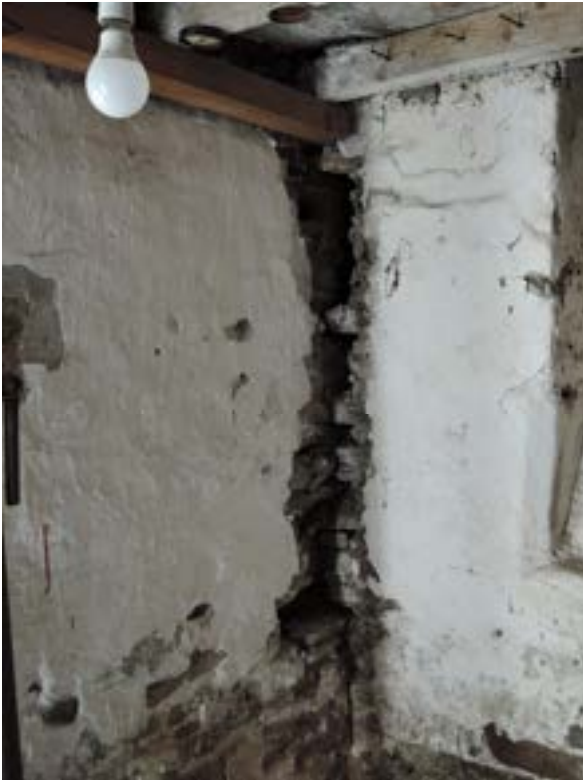
Large gap where courtyard wall is leaning away from internal buttress wall. Failed bonding/tying
