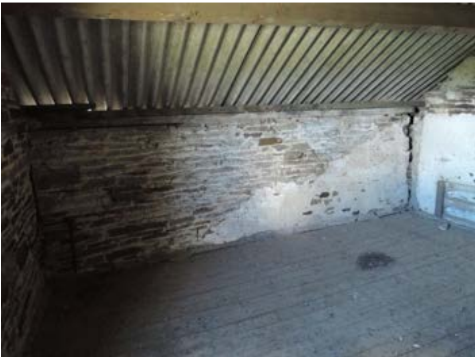
Corner cracking in wall junction indicating outward wall lean and lack of tying in
