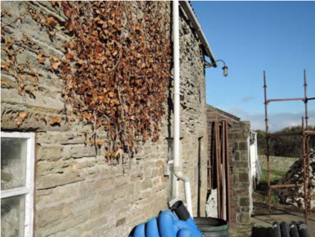
Small barn courtyard (east) wall leaning into yard abandoned first floor joist bearings (previous page)
