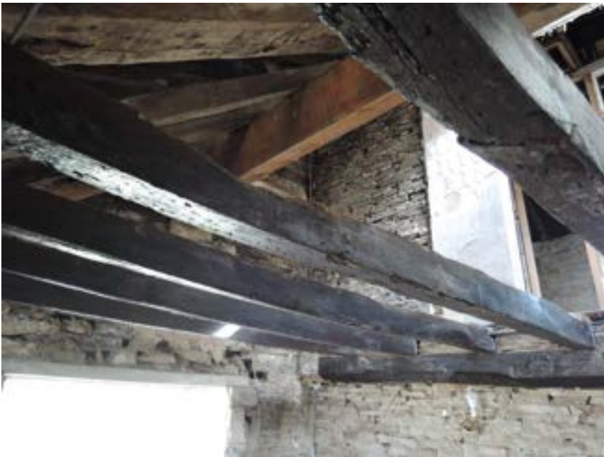
First floor (bathroom) joists over kitchen require replacement
