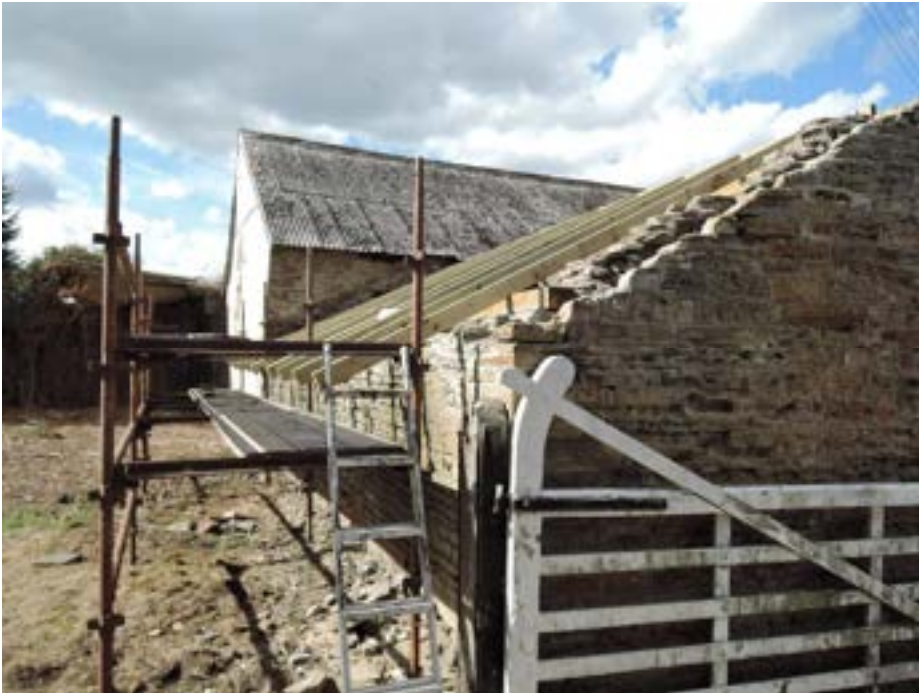
Low level shed under repair receiving new roof. Large barn in background.
