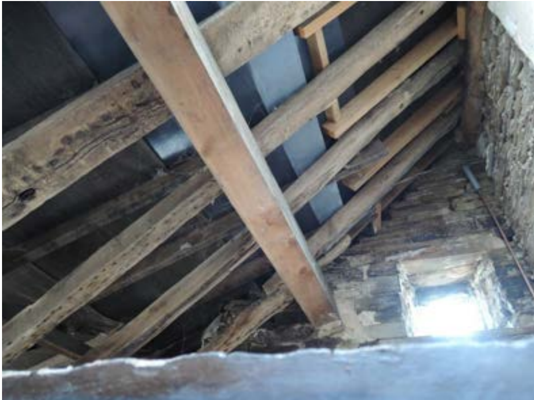
Roof over OK but to be replaced with new storey
