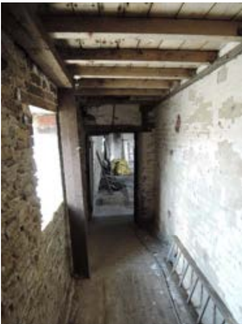
Corridor small barn. Secondary timber propping rescuing reduced bearings from outward leaning west wall.
