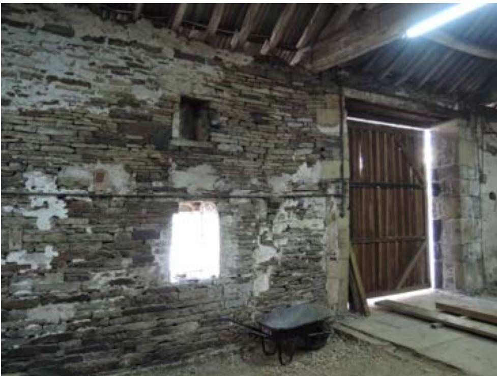
Courtyard wall and main door. Local settlement under truss left of large door. Foundation may need strengthening with local underpinning
