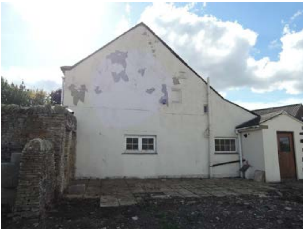
Northeast gable. Tired and peeling paint/render but no major cracks or bulging apparent.
