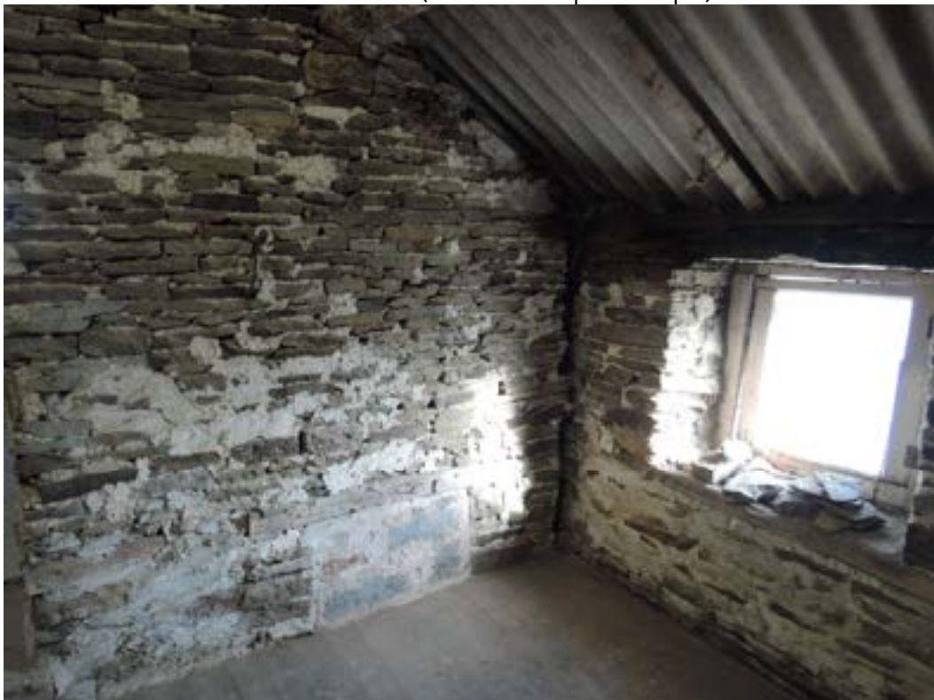
Small barn 1st floor west wall leaning out no bonding/tying to cross wall (large gap)
