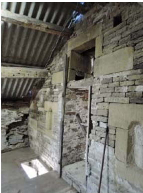
1st floor small barn. Pronounced lean of gable wall of large barn. Take down and rebuild
