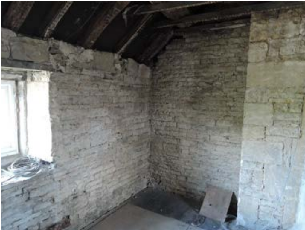
Garden side bedroom wall. Loose stones at head need looking at. Replace timber lintel.
