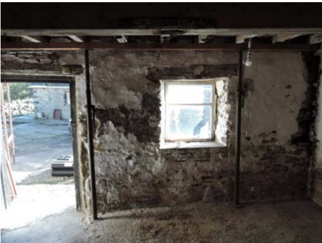
Outward leaning wall has released 1 st floor joist ends which are now only supported on a makeshift timber bearer and acrows. Failed/absent wall internal wall buttress bonding full height (far right side of picture)
