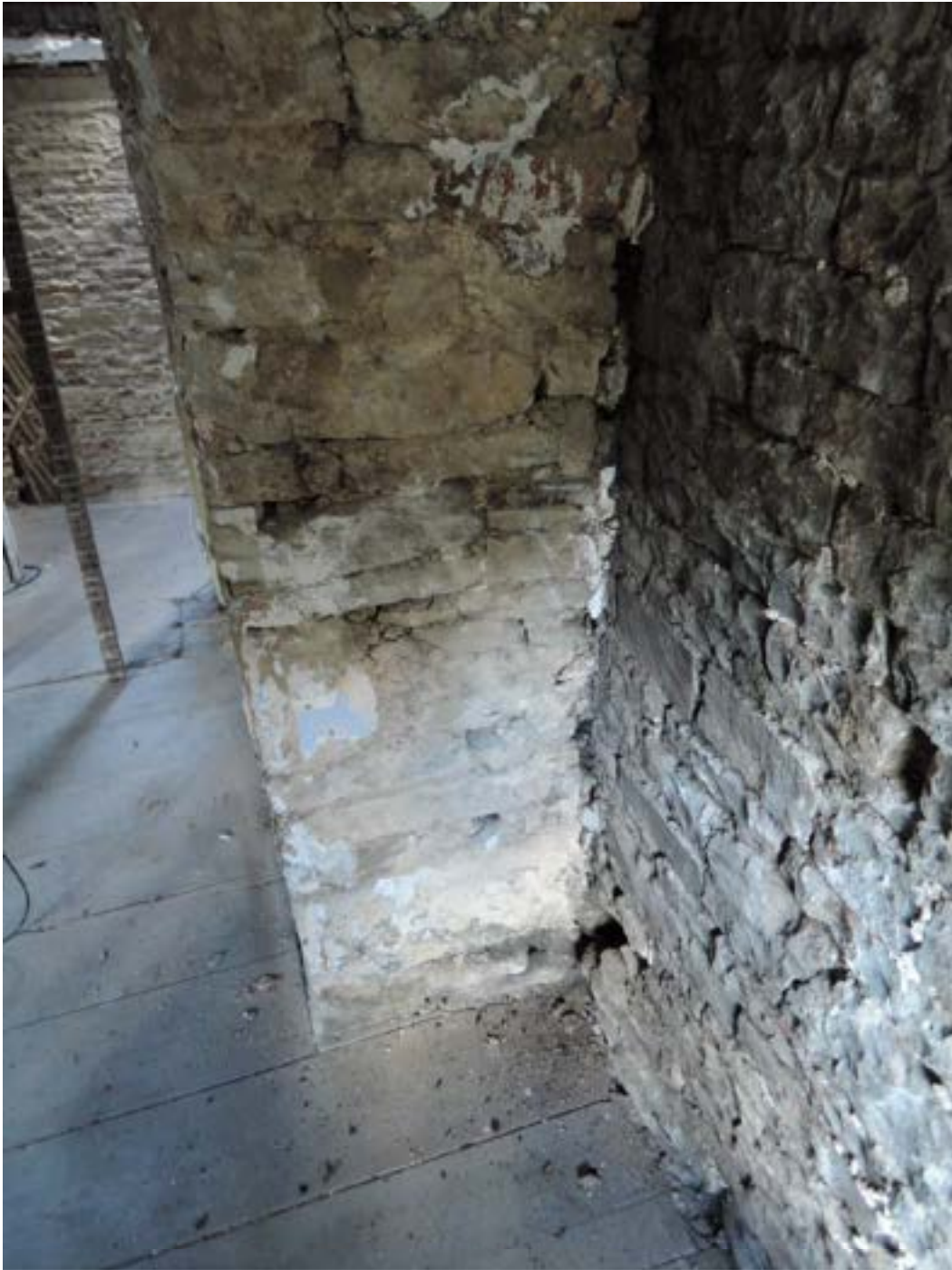
Stone flue right hand side. No bonding into wall
