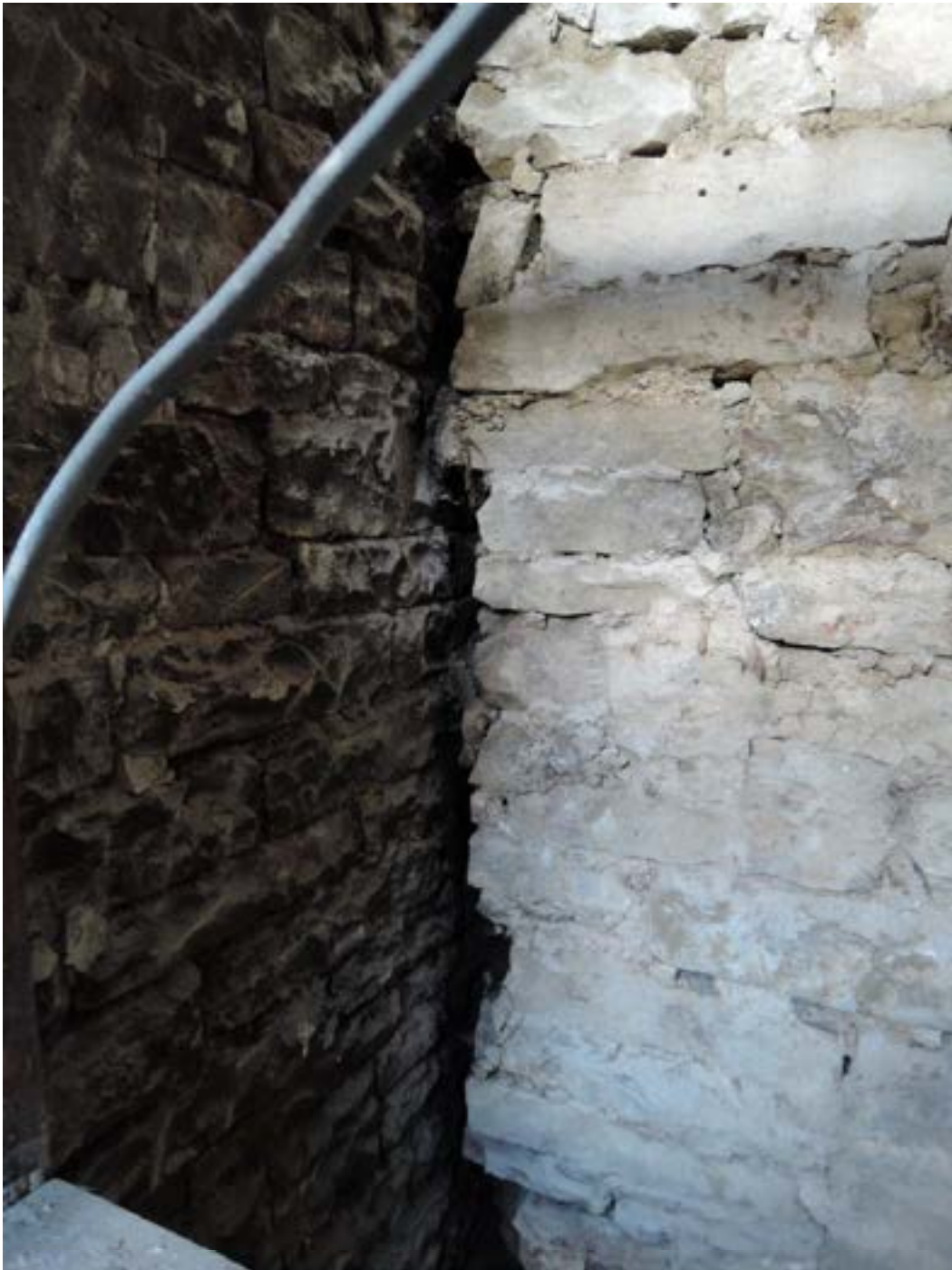
Stone flue left side not bonded into wall
