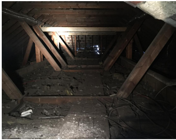
Plate 9. Loft void L1, facing south. Gaps between tiles shown on the south pitch of the hip roof.
