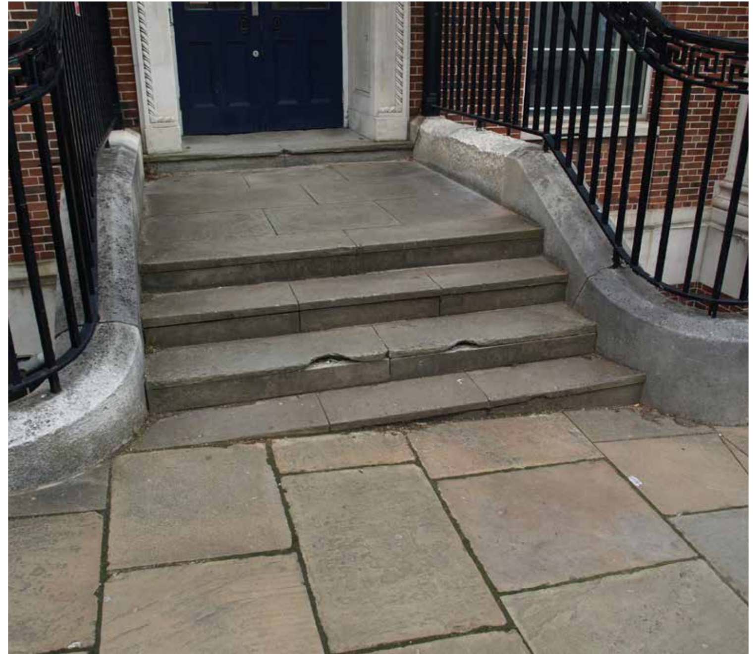
ABOVE: Stone steps and balustrade of building side southern entrance, facing north.
