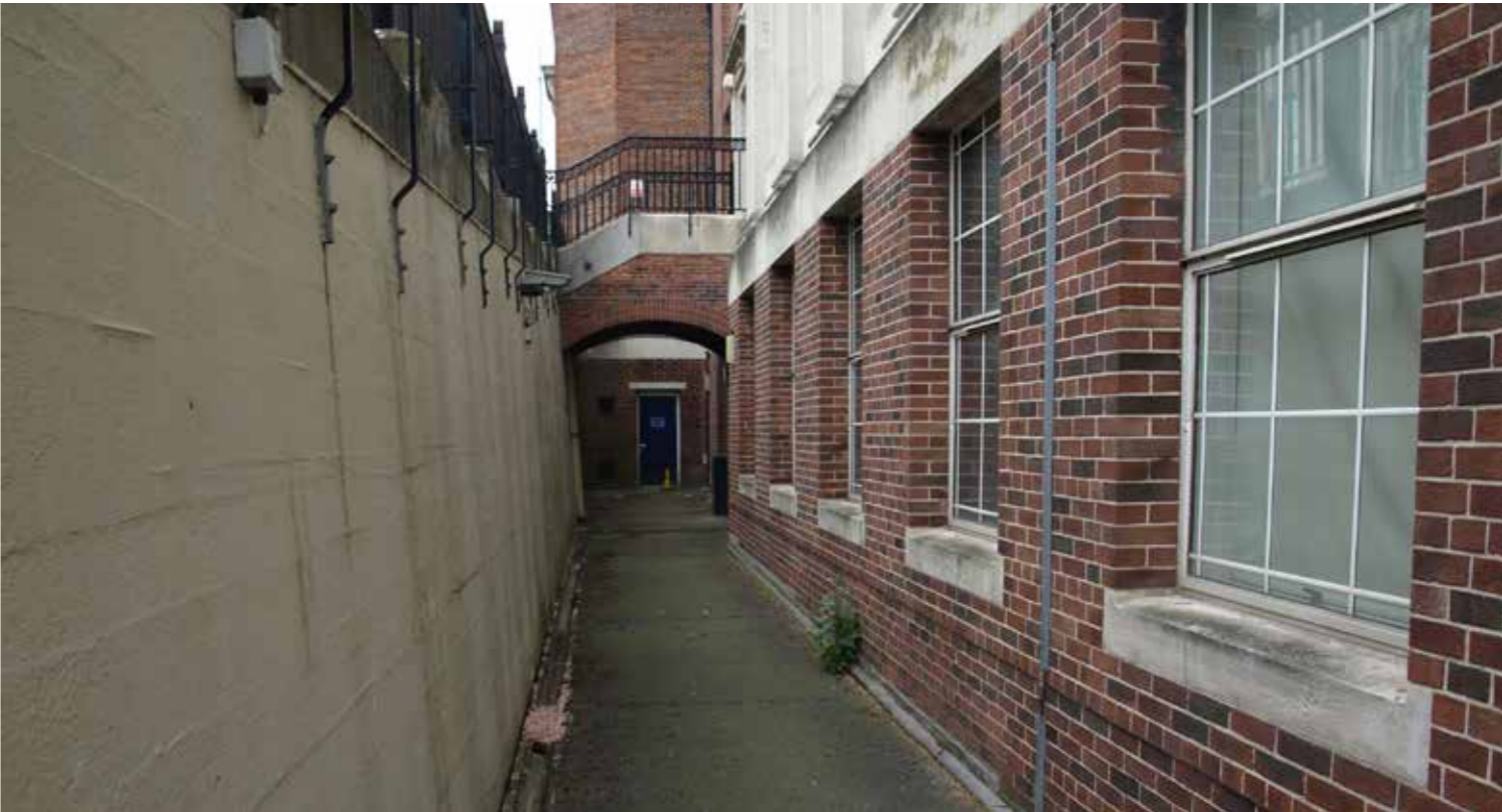
ABOVE: Arch link bridge of building side southern entrance, taken at Level 01 facing west.
