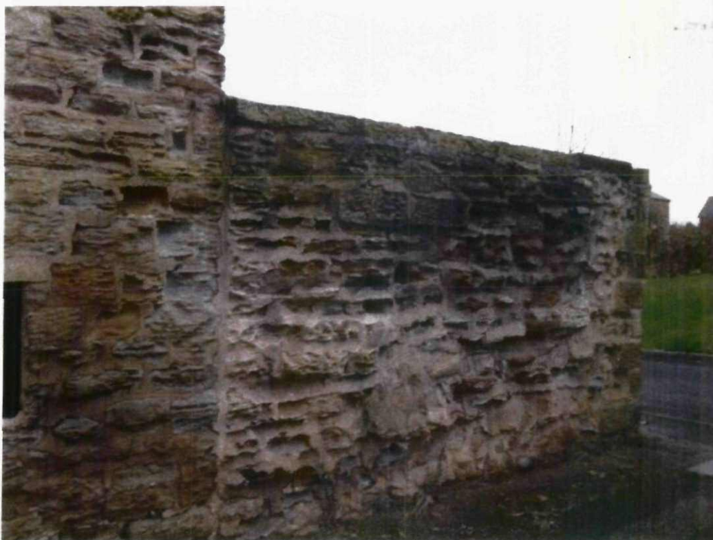
Photo 6- Outhouse wall to be rebuilt adjacent gable to 1 Old Row
