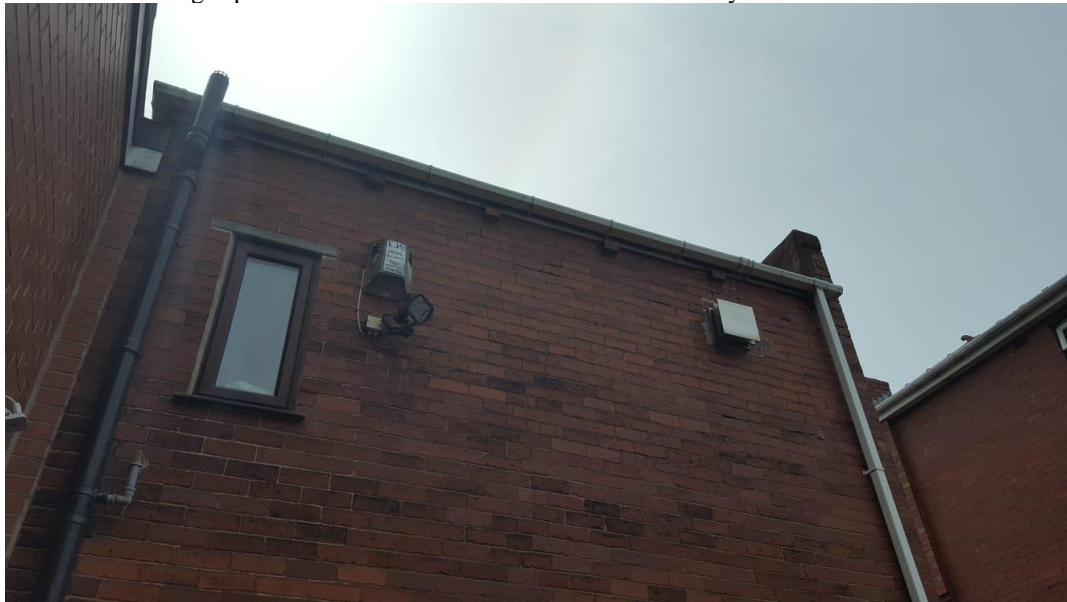
Rear elevation showing the adjoining property having been previously extended at both ground and first floor level at the rear.
