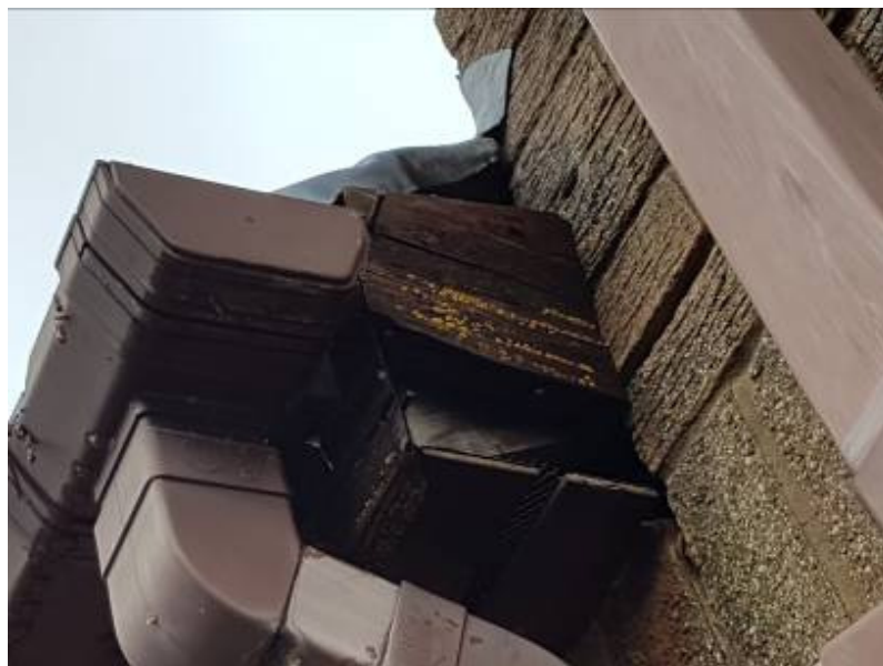
Photograph 1a Minor gap at soffit board
