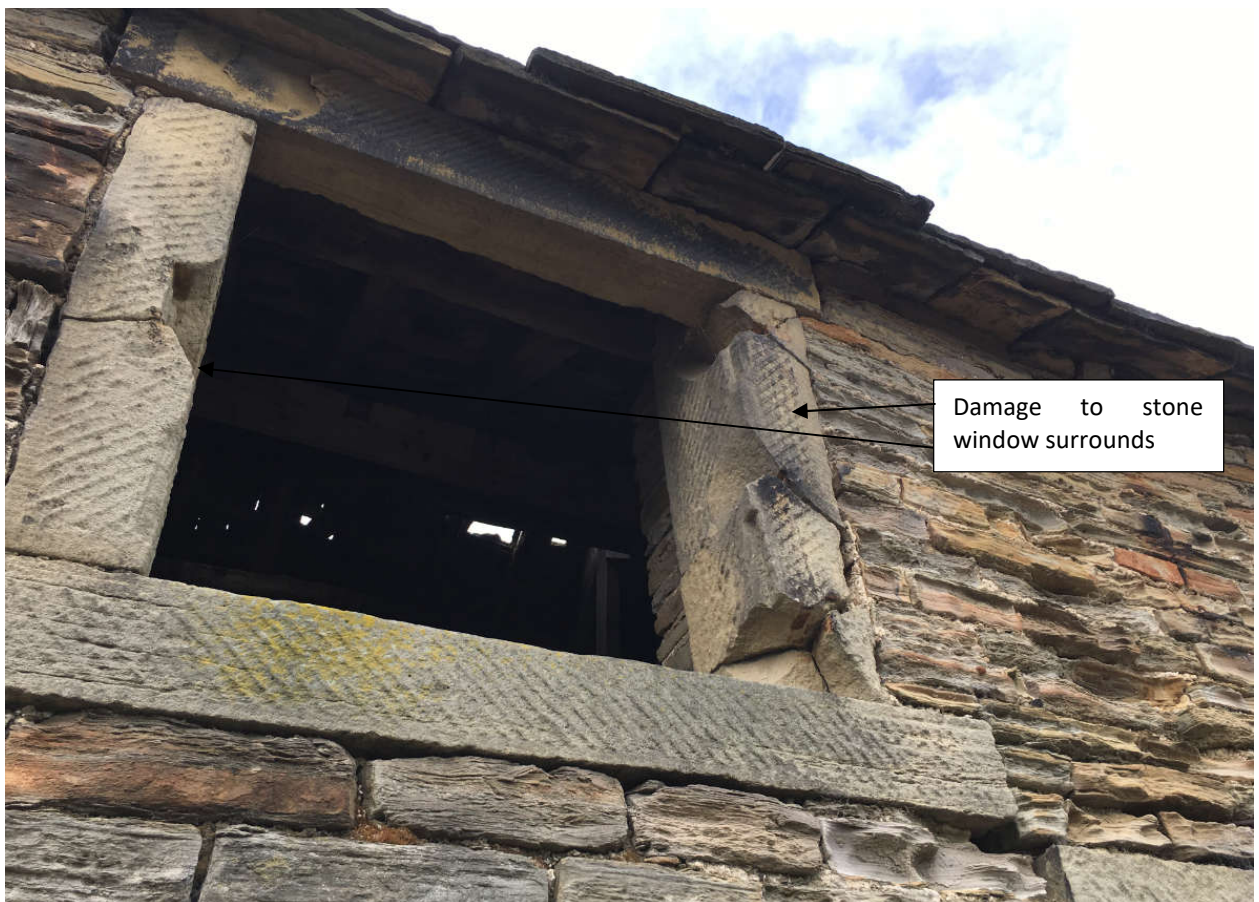
18. Damaged Window Surrounds to Building 4
