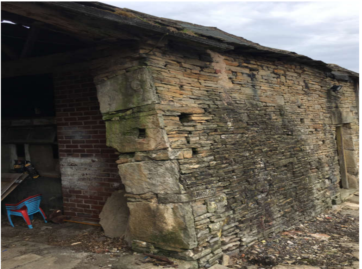
8. Leaning Wall to Building 1 (RHS of opening)
