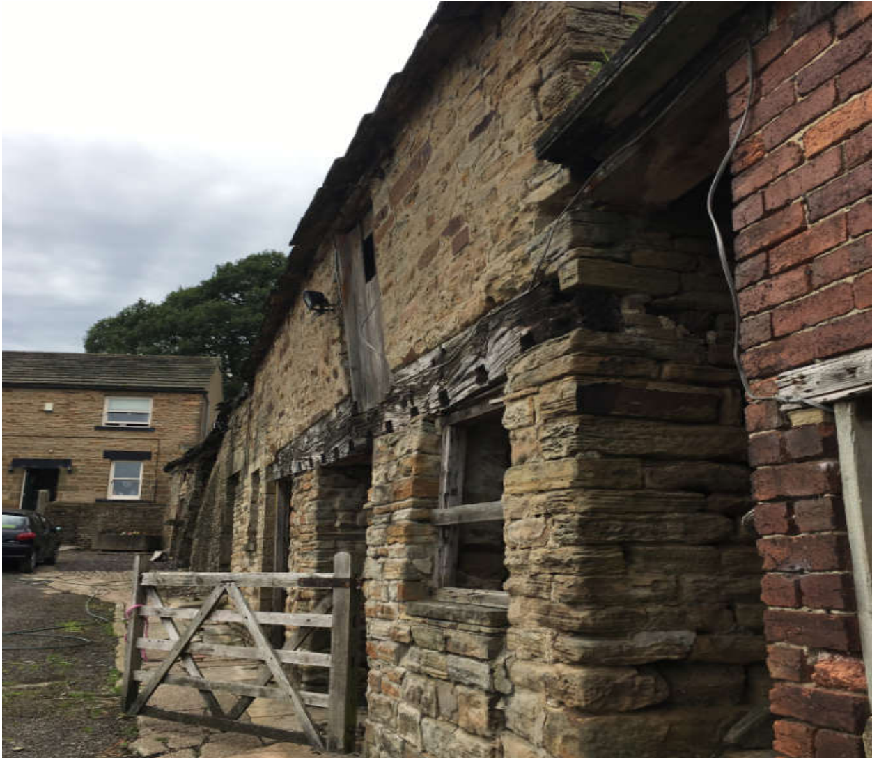
9. Leaning Wall and Timber Lintel to Building 3
