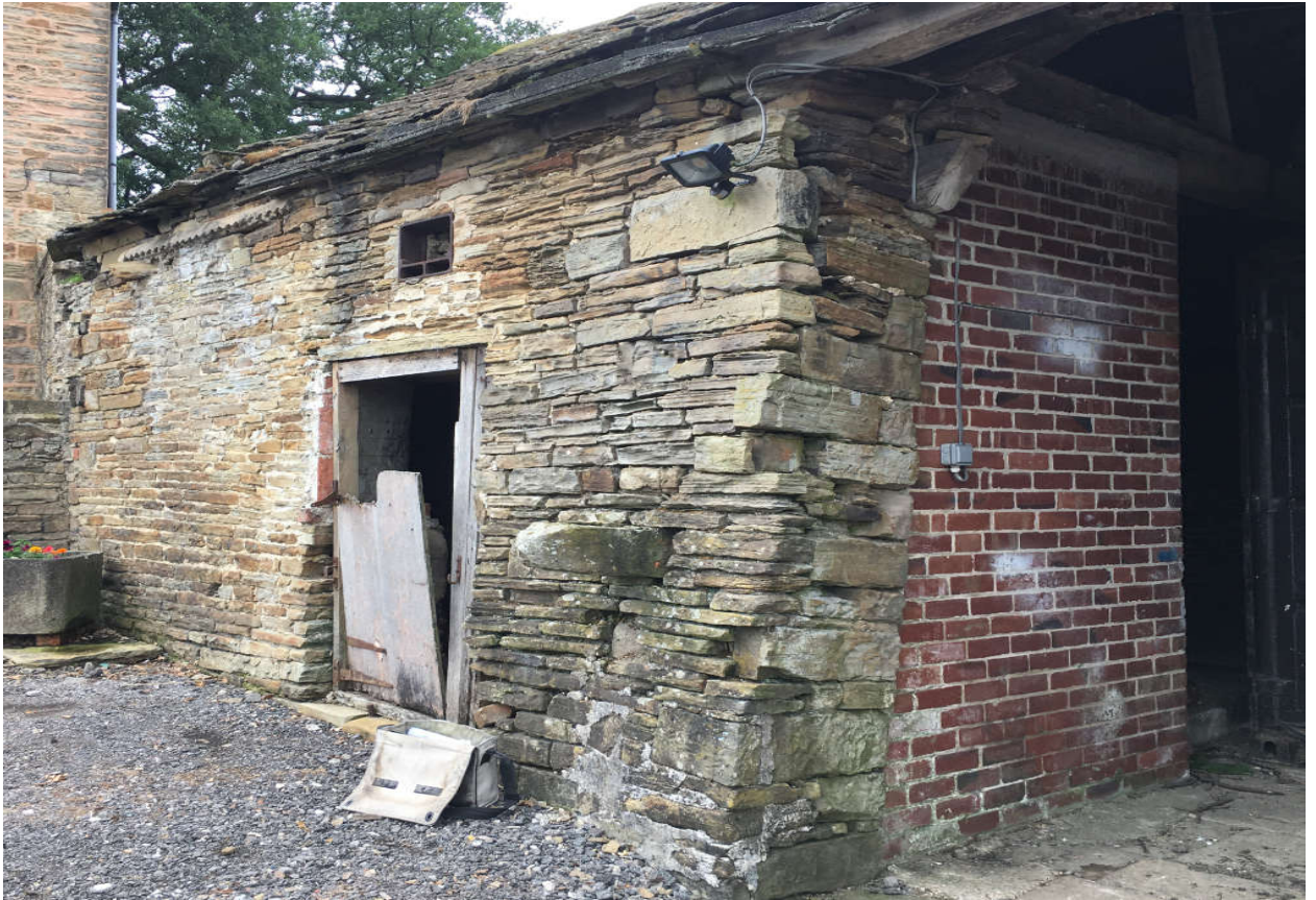
7. Leaning Wall to Building 1 (LHS of opening)
